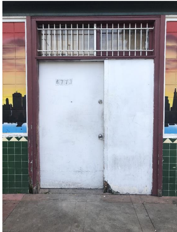
Original storefront entrance opening with replacement door and surround, 4773 Mission Street, January 2020.
