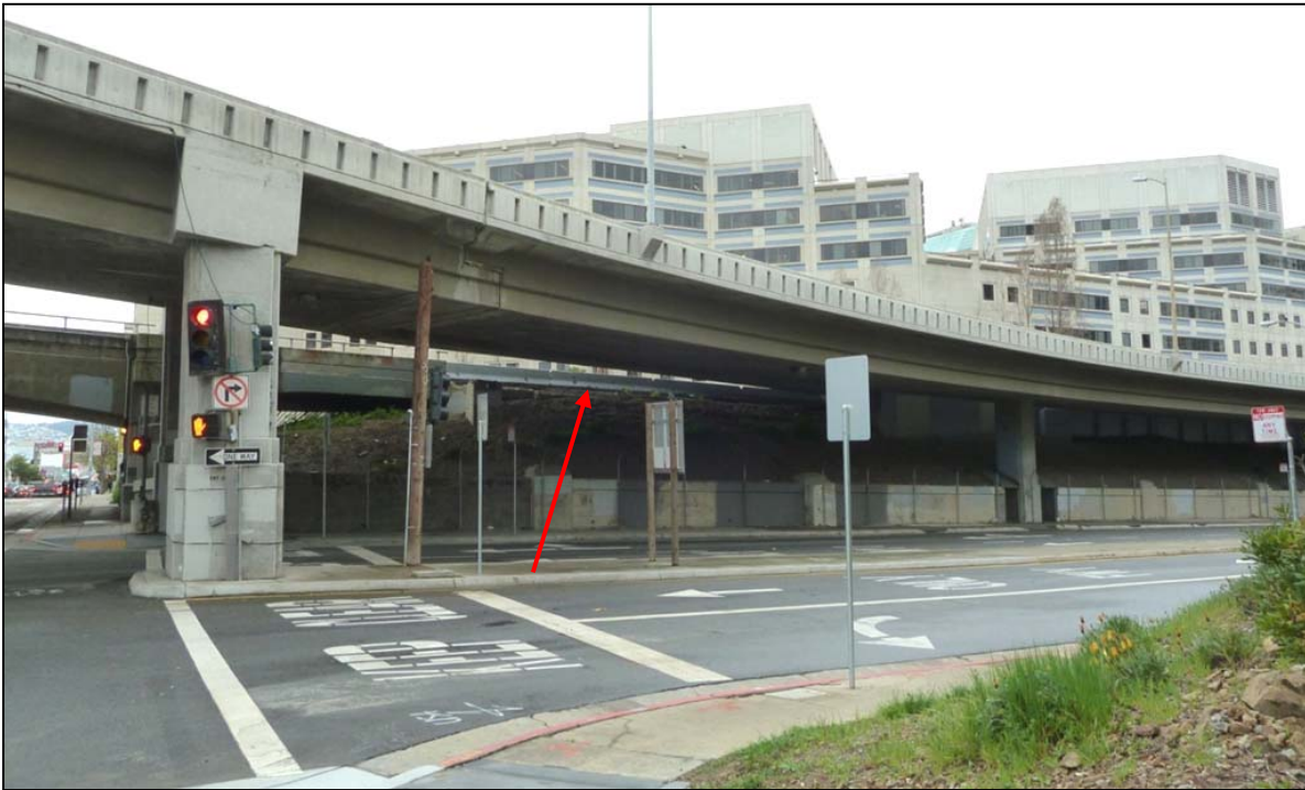
Photograph 2: Portion of the former Transbay Terminal Bus Ramp that passed through the Project Area prior to its demolition. Fremont Street exit ramp in foreground remains and is not historic. Camera facing southwest, JRP April 2011.
