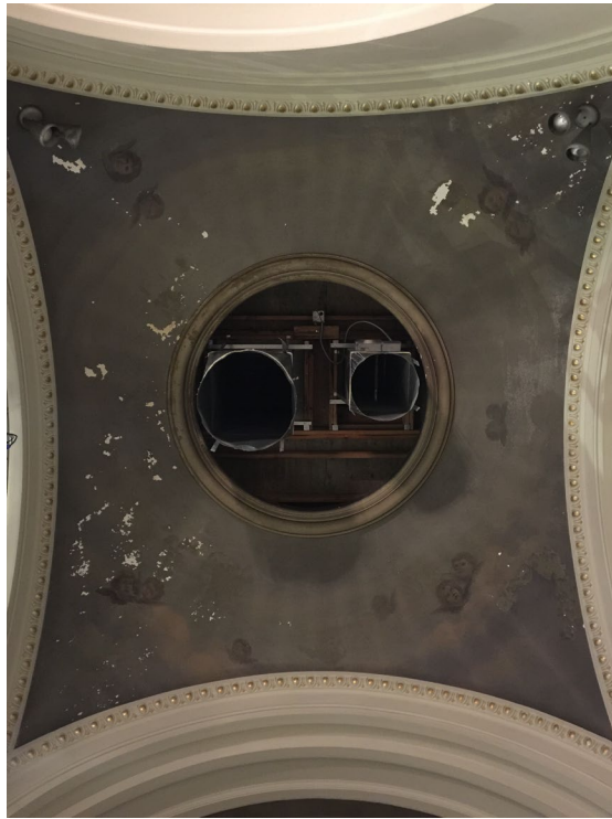
View of mechanical equipment located in the ceiling of the eastern side aisle.
