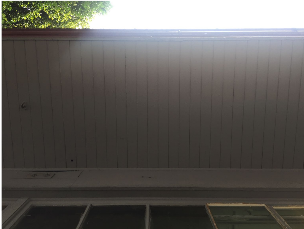
Soffit above storefront at 2857 24 th Street, December 2018.
