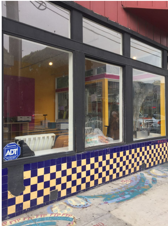
Detail of bulkhead, storefront windows, and raised window display areas at the interior, 2851 24 th Street, view southwest, December 2018.
