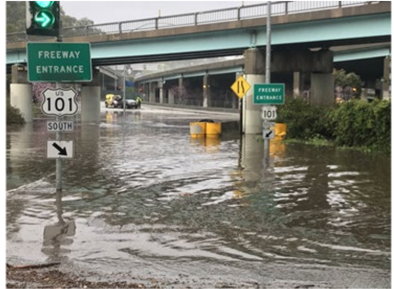
Flooding in Lower Alemany Area
