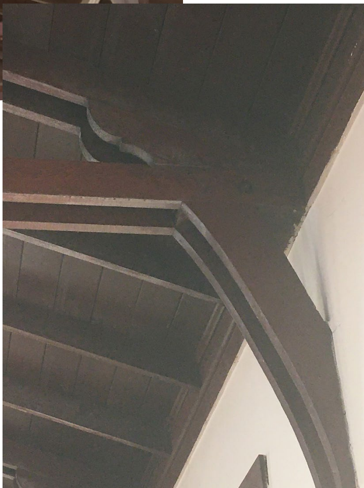
St. James Presbyterian Church, details of ceiling, trusses, and brackets in sanctuary, 2022 Source: San Francisco Planning Department
