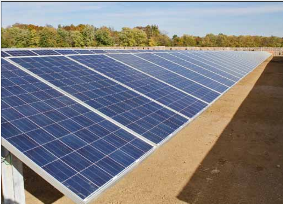
The "Indy I" Solar Array depicted is one of three utility-scale solar projects owned by Dominion Energy Resources—these projects represent a combined 28.6 MW of solar power in Indianapolis.
