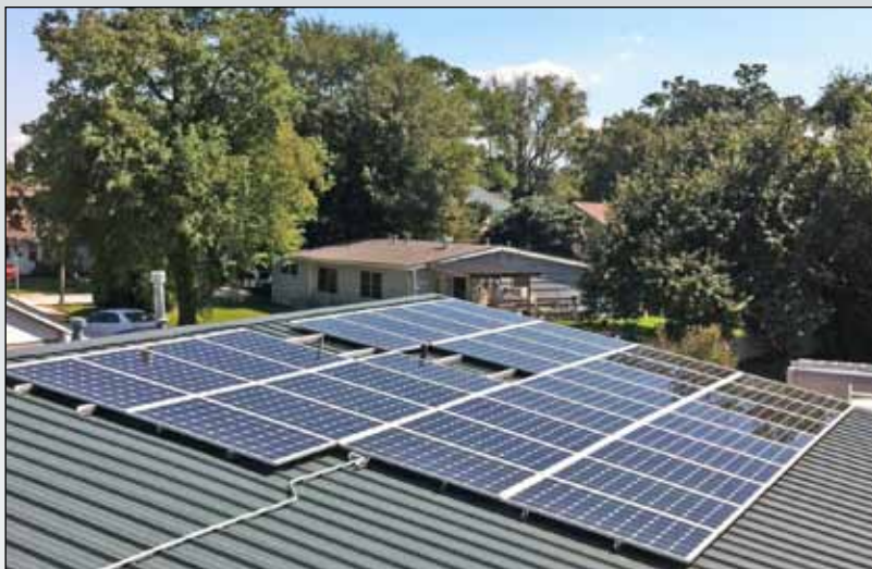
A rooftop solar installation generates clean energy in New Orleans.
