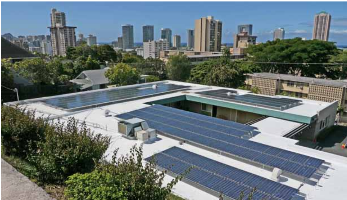
Solar panels on the roof of the non-profit Easter Seals Society building with downtown Honolulu in the background.
