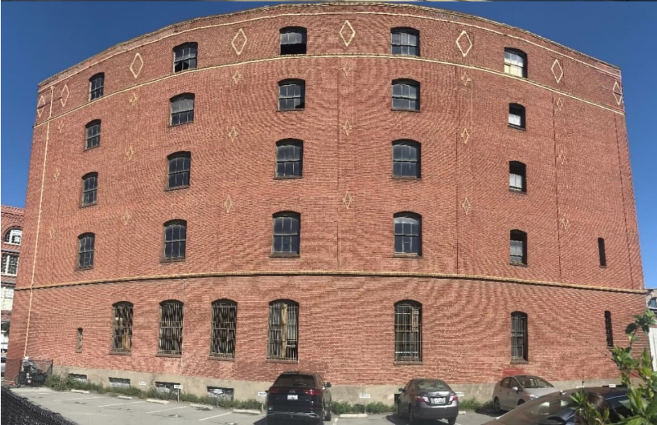
Above: North façade. Architectural Resources Group, July 2019 Below: Northwest façade Planning Department Staff, August 2021
