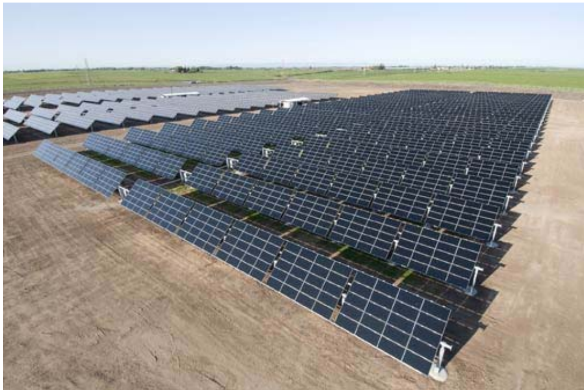
At Grade – Single Axis Tracking
