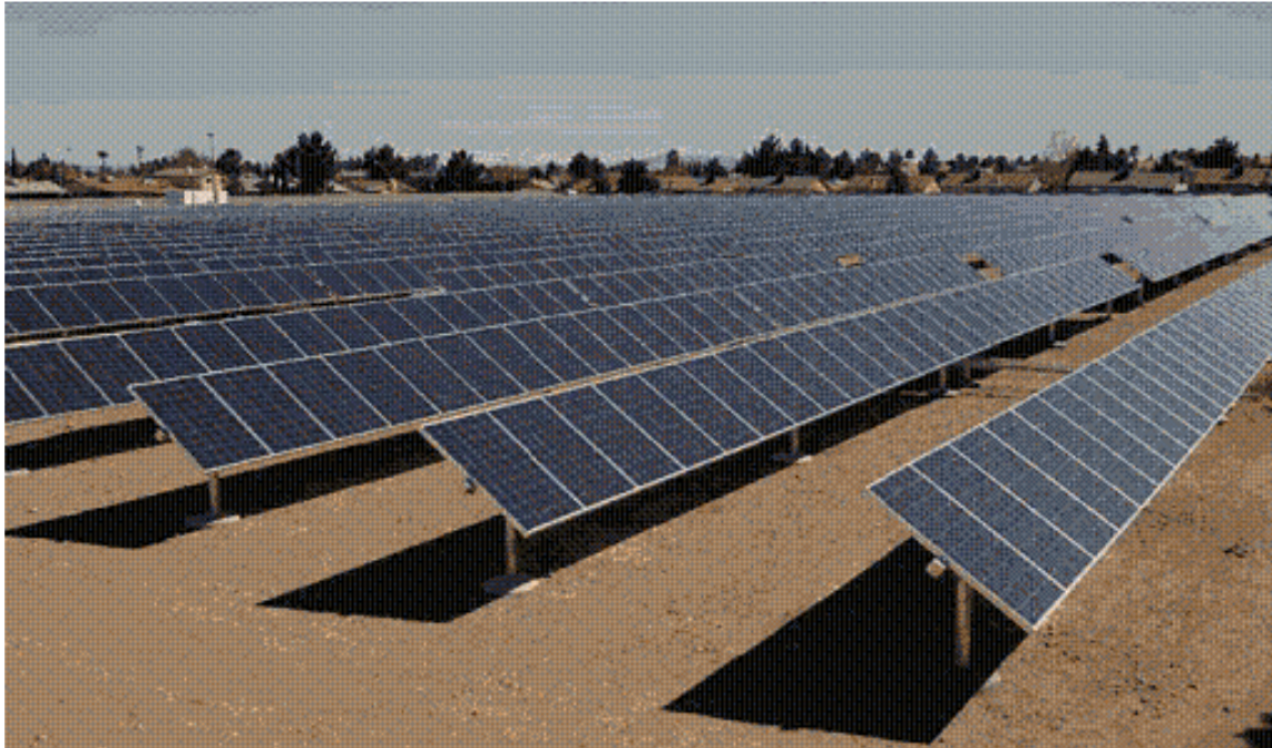
At Grade – Fixed Tilt
