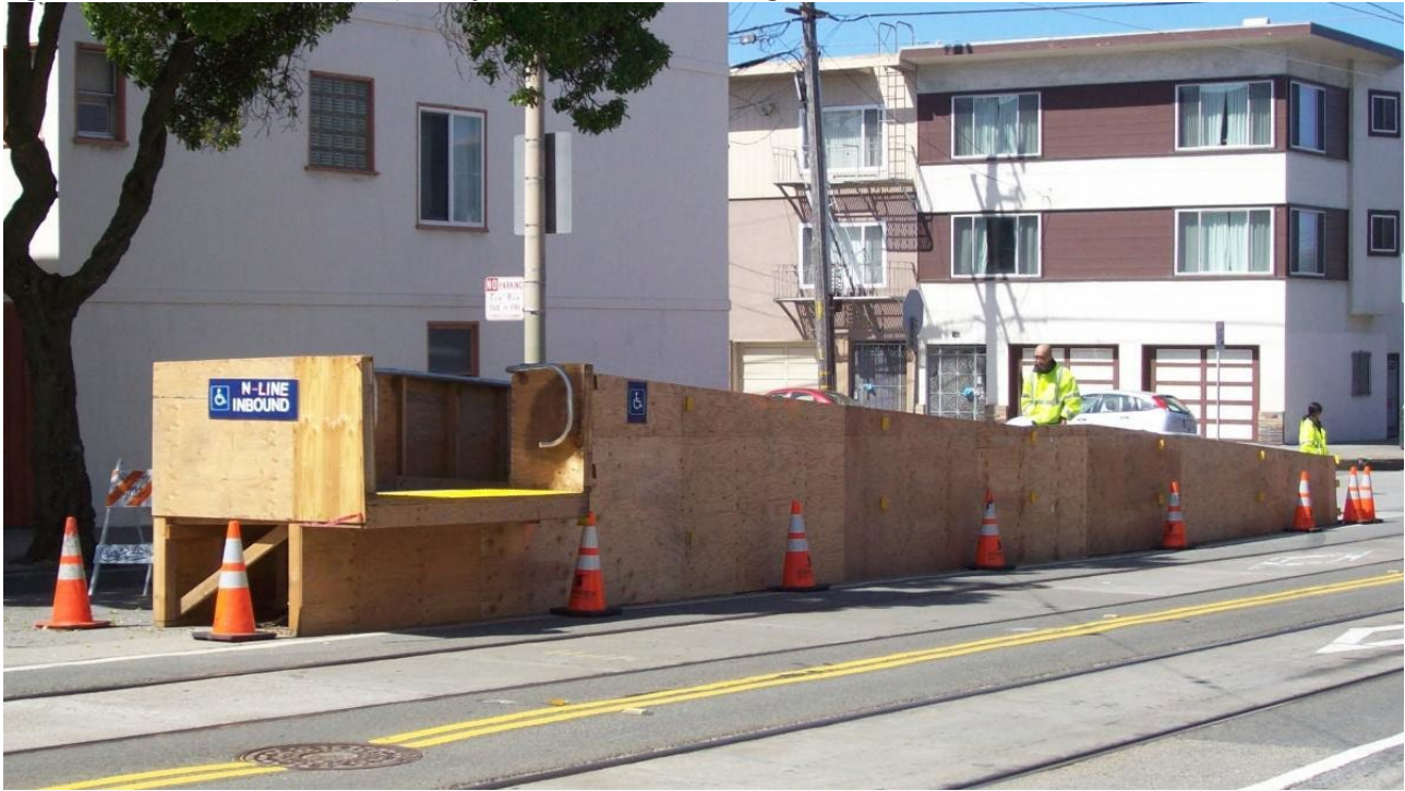
Figure 3: Example of a Temporary Accessible Boarding Island
