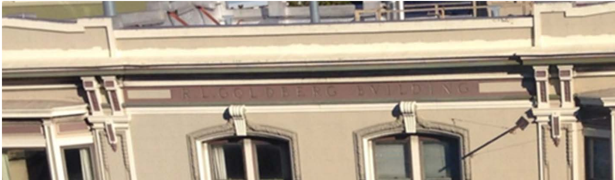
Figure 1 "R. L. Goldberg Building" is incised with Roman italic letters in the cornice of the west façade.
