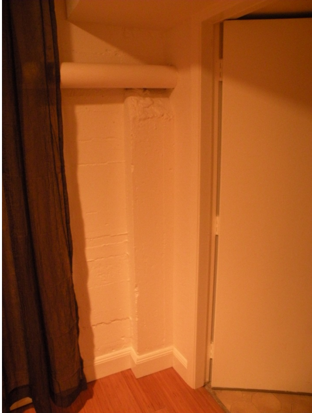
Figure 45 Impressions on the basement wall reveal that the foundations are cast board-formed concrete.
