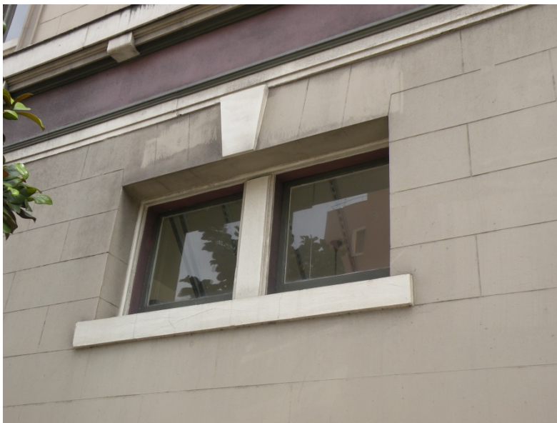
Figure 19 Pair of square raised windows with keystone and incised stucco in imitation of stone set high on the Oak Street elevation's first story.
