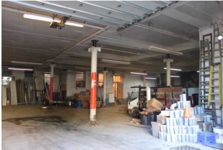
FIGURE 13. CHURCH: BASEMENT SHOWING GUTTED CONDITION, 2015.
