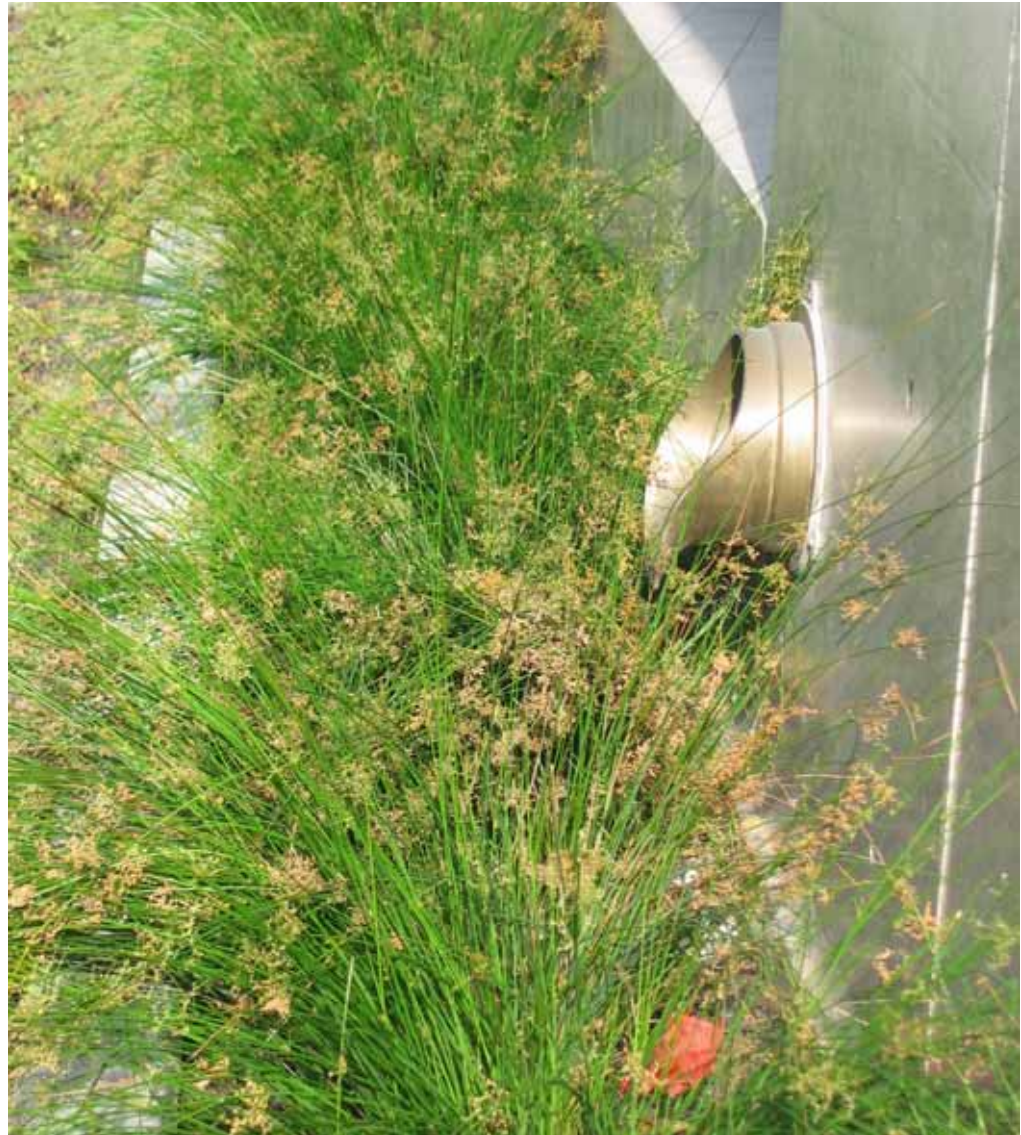
An interior roof drain discharges to a vegetated swale in Emeryville, CA. This properly designed and permitted stormwater facility is an “approved alternate location” for stormwater discharge.
