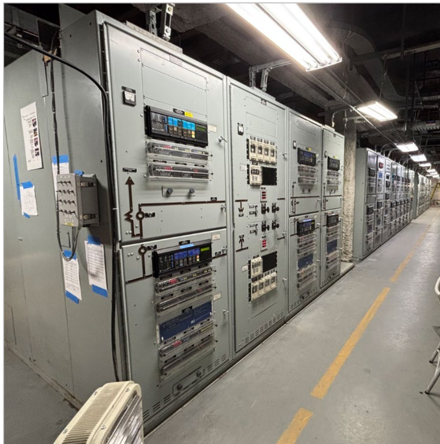
Figure 2. 12 kV Switchgear at Mission Substation.
