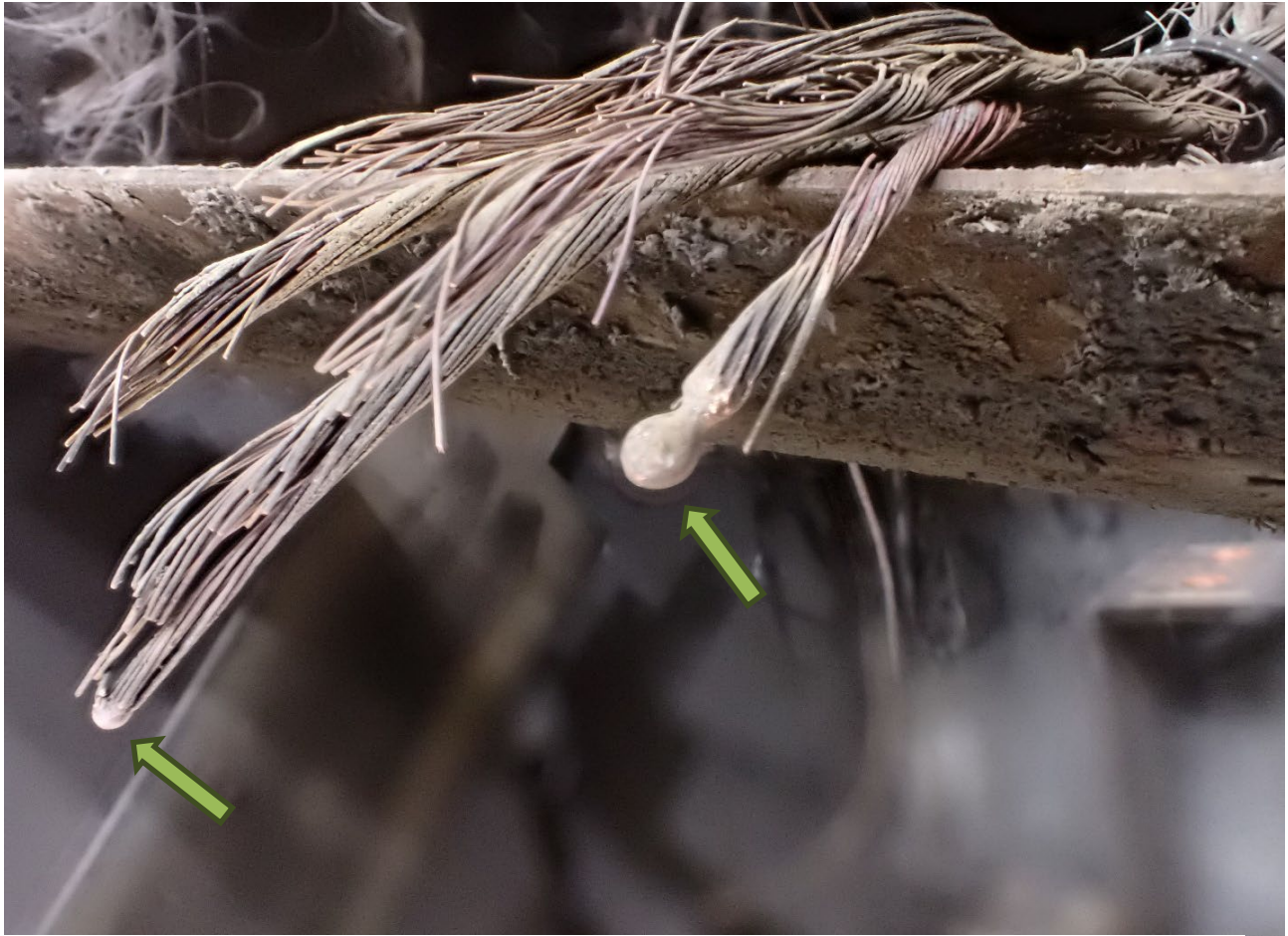
Figure 25. Evidence of electrical arcing on CT wires (green arrows).
