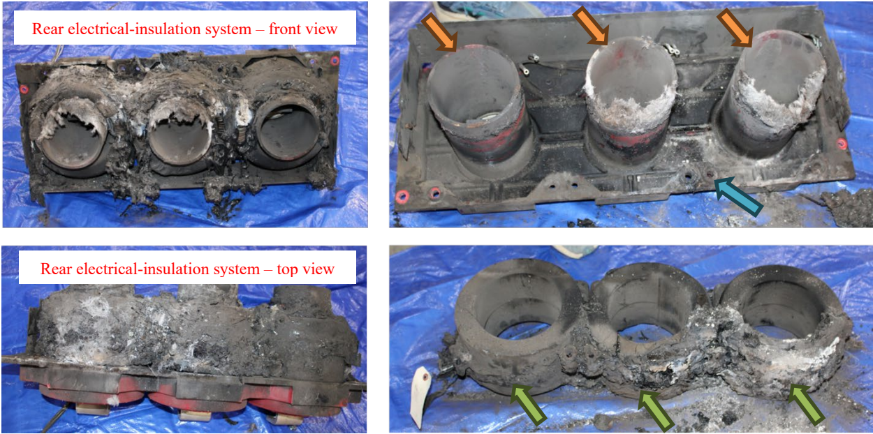
Figure 27. Cubicle’s rear electrical-insulation system and components (lower row) showing CT insulating tubes (orange arrows), busbar penetration wall (blue arrow), and current transformers (green arrows).
