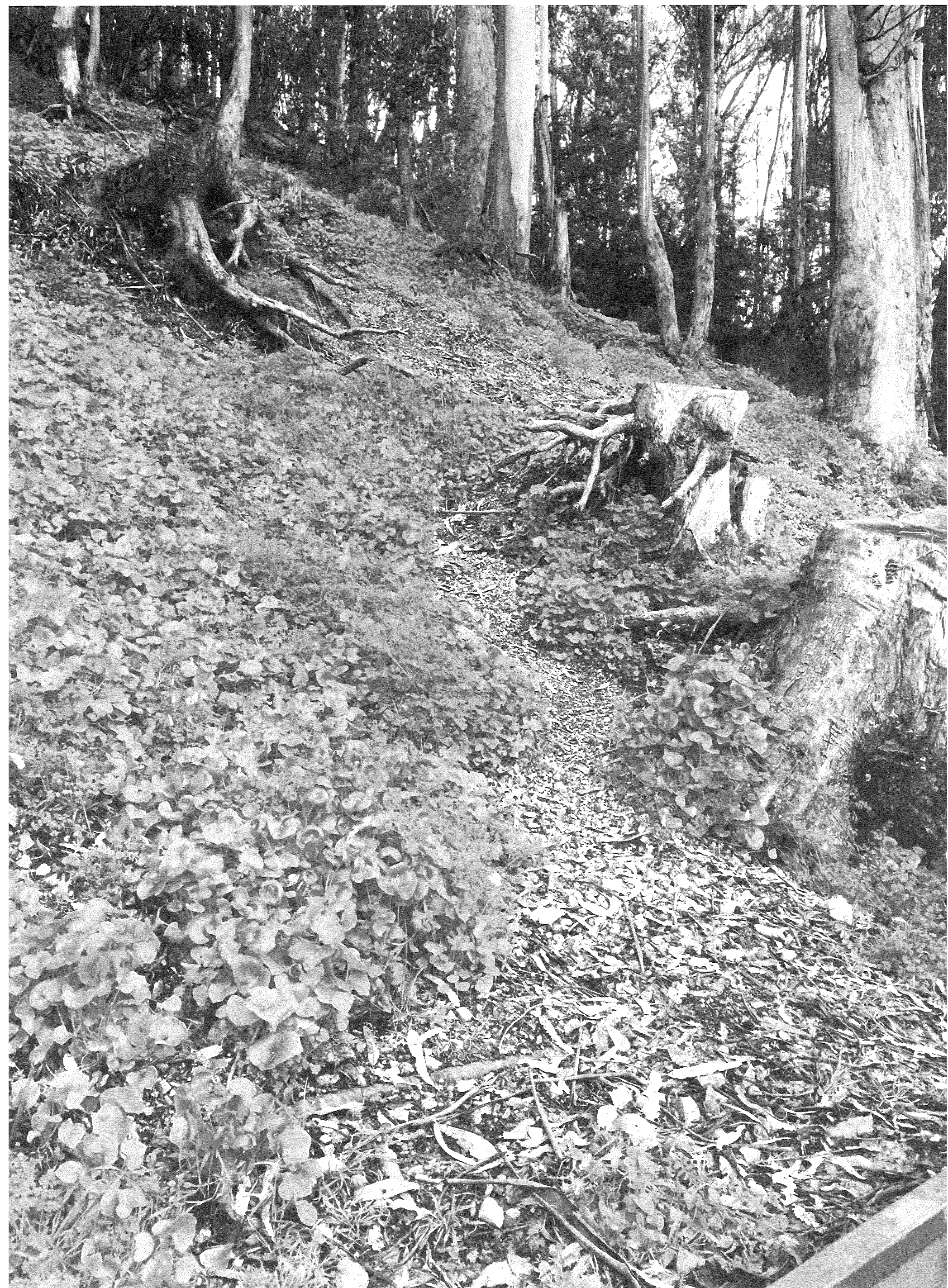
GLEN PARK WHERE STUMPS ARE, there is nothing to Absorb water dead Stumps = EROSION
