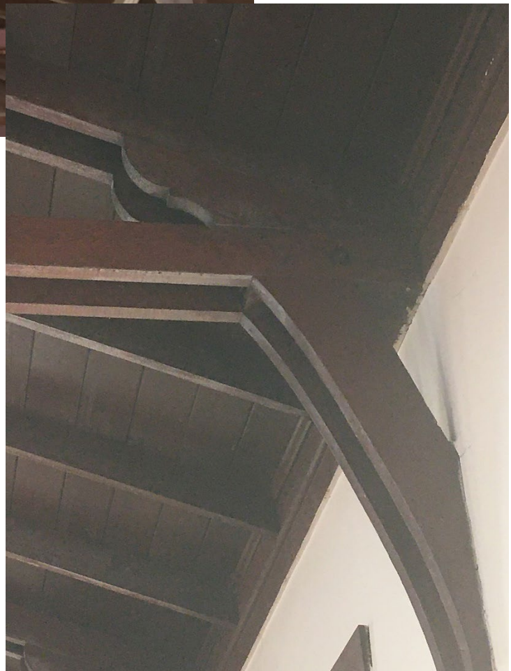
St. James Presbyterian Church, details of ceiling, trusses, and brackets in sanctuary, 2022 Source: San Francisco Planning Department
