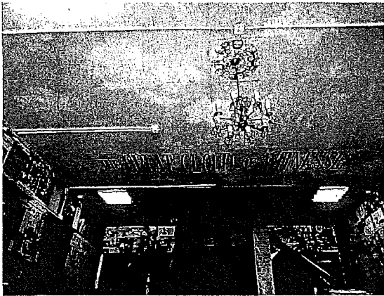
Figure 7: Painted ceiling appears to be in good condition with no flaking or chipping paint.
