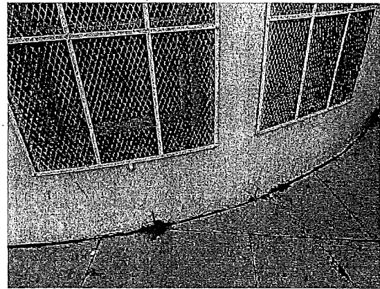
Figure 4: Biogrowth at base indicates possible inadequate drainage.
