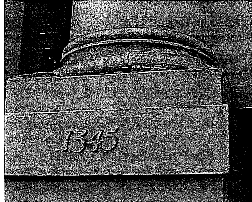
Figure 2: Cracking of concrete column at base.
