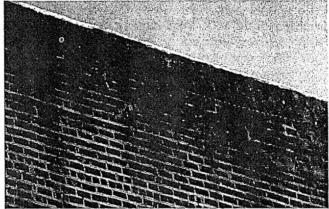
Figure 5. East elevation at roof parapet; note bio-growth and discoloration to be addressed prior to rehabilitation work.
