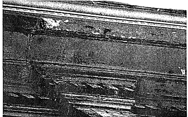
Figure 4. Cornice; conditions noted as typical.
