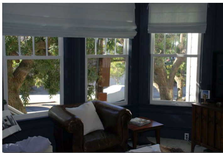
Equipment cabinet for a Personal Wireless Services Facility in front of a residential bay window. Many of the larger cabinets feature cooling fans that may be bothersome to residents.
