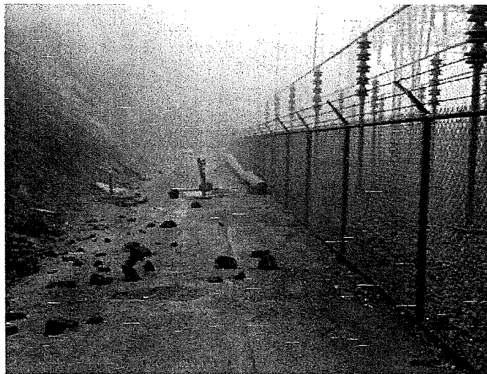
Figure 1-2: Rockfalls at Slope along South Edge of ISY (August 27, 2013)
