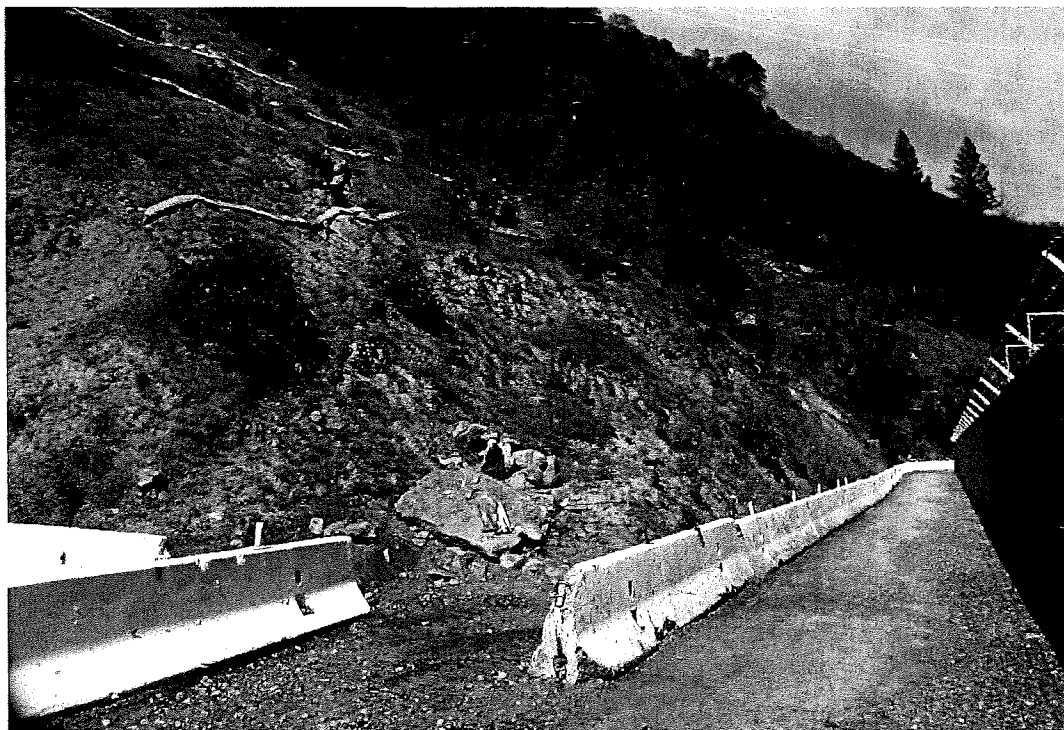
Figure 2-7: Slope Debris from Raveling Slope alongside Access Road on South Edge of ISY (May 2, 2014)
