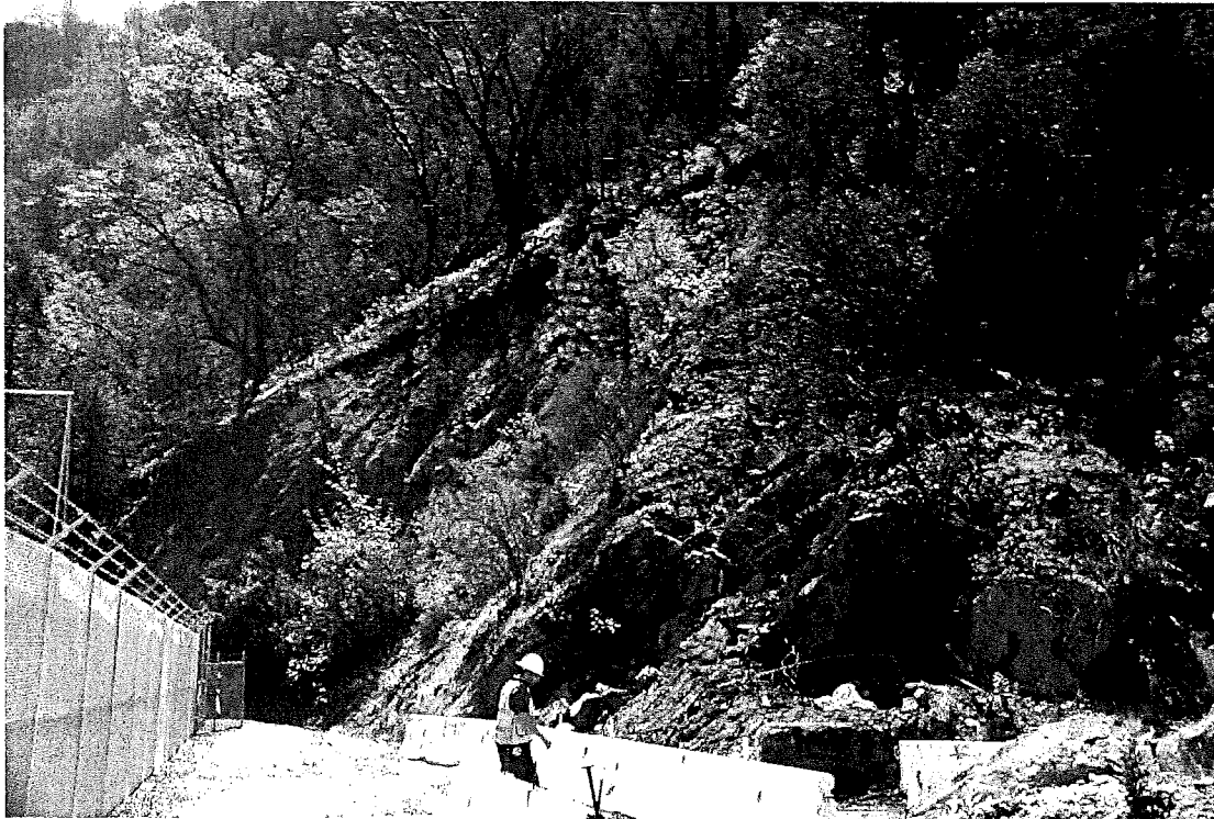
Figure 2-5: Work Area 1 – Active Slope Failure at East End of ISY (May 2, 2014)
