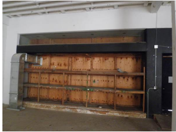
Figure 11. 113-115 Steuart Street, view of altered ground floor from the interior (boarded on exterior). Source: Page & Turnbull, August 2013.
