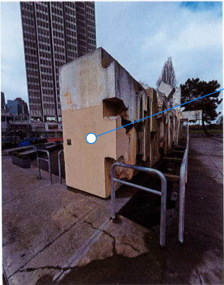
Photo 4. Rear wall – no reinforcing steel was found.
