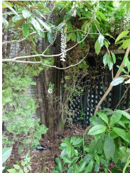
Figure 12: Brick wall (left) and building's north façade (right) showing the lack of accessibility to the east façade, facing southeast.
