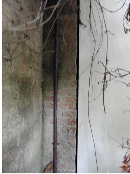
Figure 8: Perimeter brick wall (left) and building's south façade (right) showing the lack of accessibility to the west façade, facing north.
