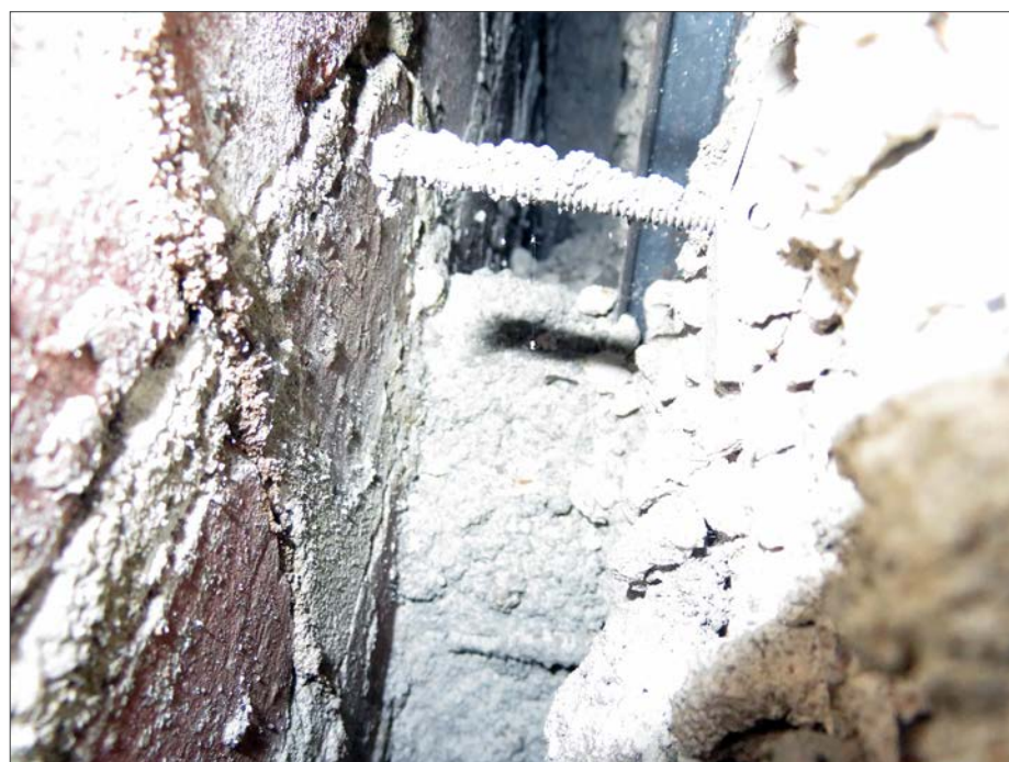
Probe 5, looking to the right and slightly down. Note the wad of mortar in the void at the furring channel. The toggle bolts are part of the handrail installation.
