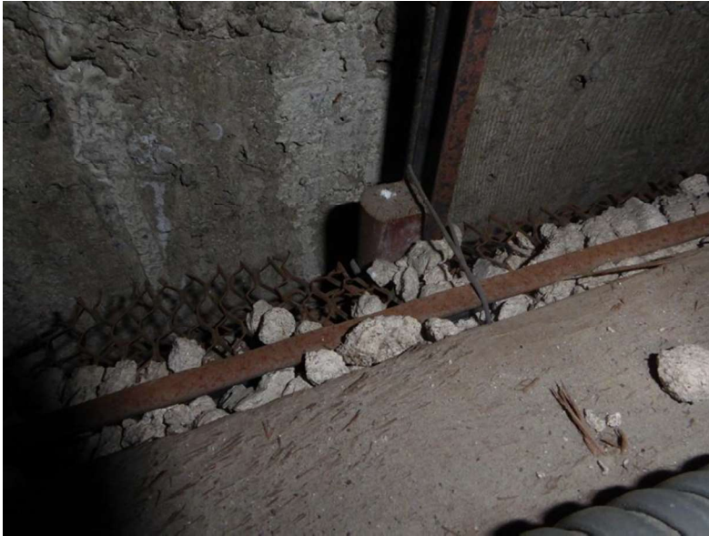
Figure 3: View looking down toward rear of fresco showing metal furring with wood nailer and attachment
