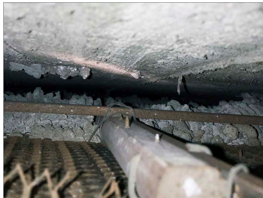
View behind Fresco 3 from above. Note the small void space and horizontal channel wire tied to the vertical furring channel. Photo by Tuan and Robinson.
