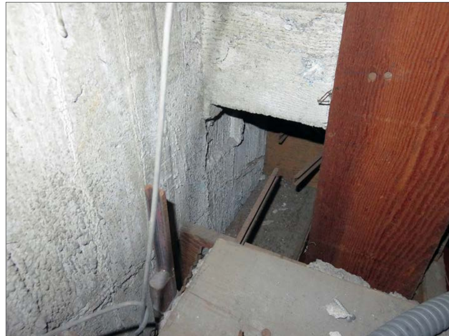
Pilaster between Frescos 3 and 4 from above. Note the board nailed to the concrete and supported furring channels of the ceiling.
