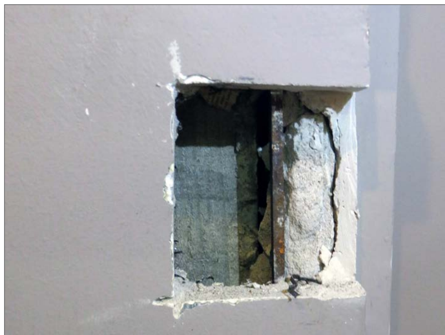
Probe 3. Note the black iron furring channel in the corner. The void space here was not filled with plaster debris, which is consistent with it being an area of repair.
