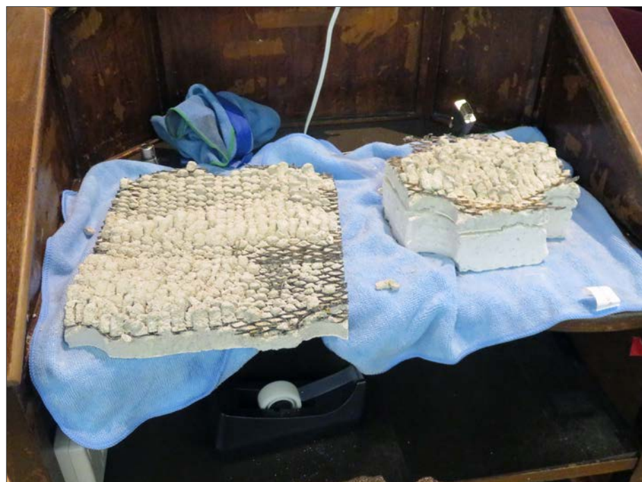
Plaster from Probe 1 and Probe 6. Note the presence of a distinct scratch coat and brown coat.
