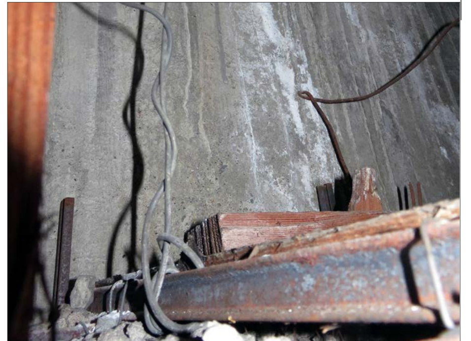
Ceiling above Fresco 7. Note the salts on the concrete from moisture infiltration and the use of the concrete form tie to hang the black iron support of the ceiling.
