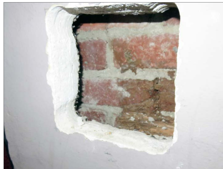
Probe 6. Note the wood block in the lower portion of the opening.
