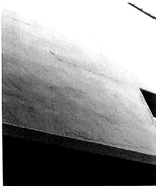
Figure 22 - Visible bulging at the crack repair on the east facade of the Annex; there is the potential here for failure in the future. Photo by Page & Turnbull
