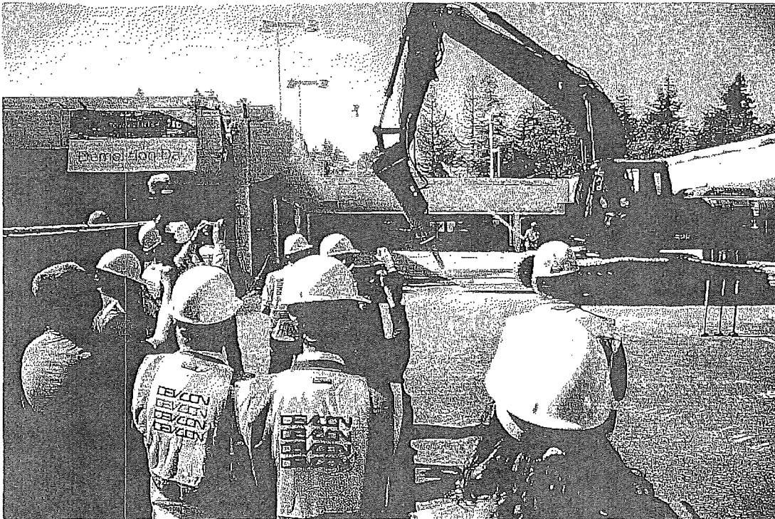
Demolition of a parking structure at the Vallco Shopping Mall began on Thursday, Oct.11, 2018, after an hour-long press conference celebrating the milestone in Cupertino, Calif. (Karl Mondon/Bay Area News Group)
