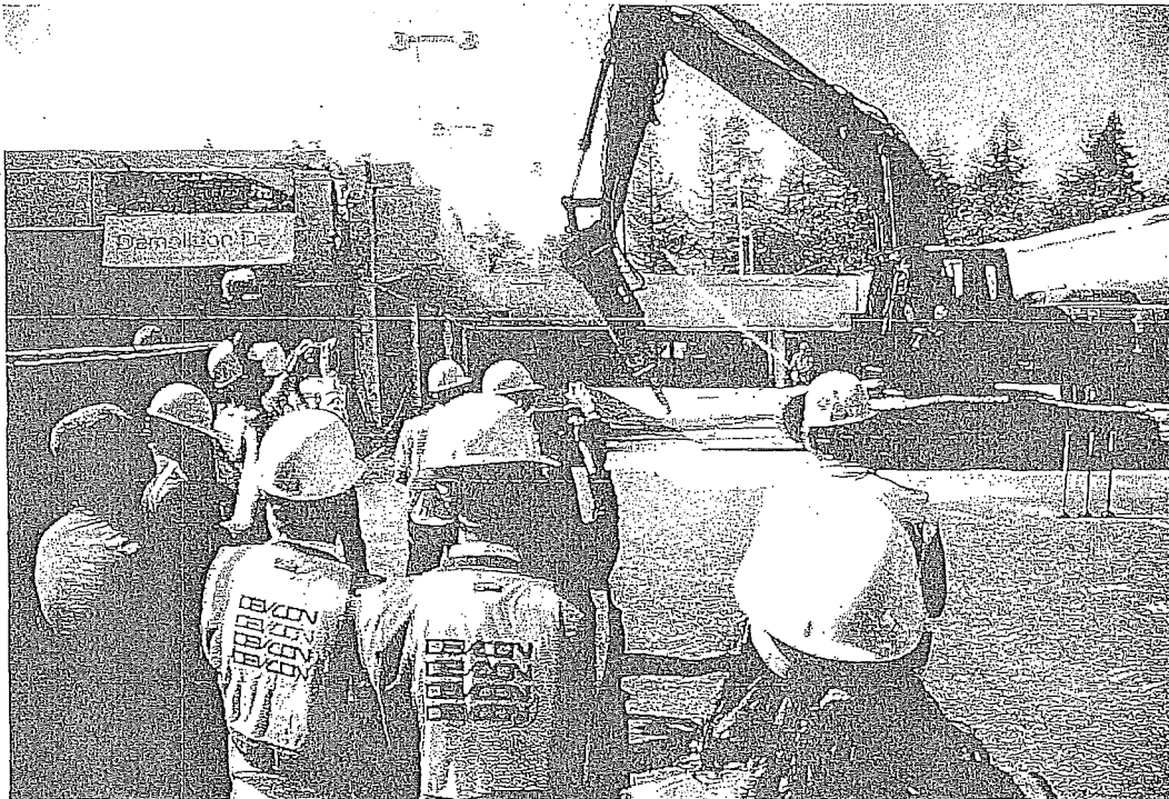
Demolition of a parking structure at the Vallco Shopping Mall began on Thursday, Oct. 11, 2018, after an hour-long press conference celebrating the milestone in Cupertino, Calif. (Karl Mondon/Bay Area News Group)
