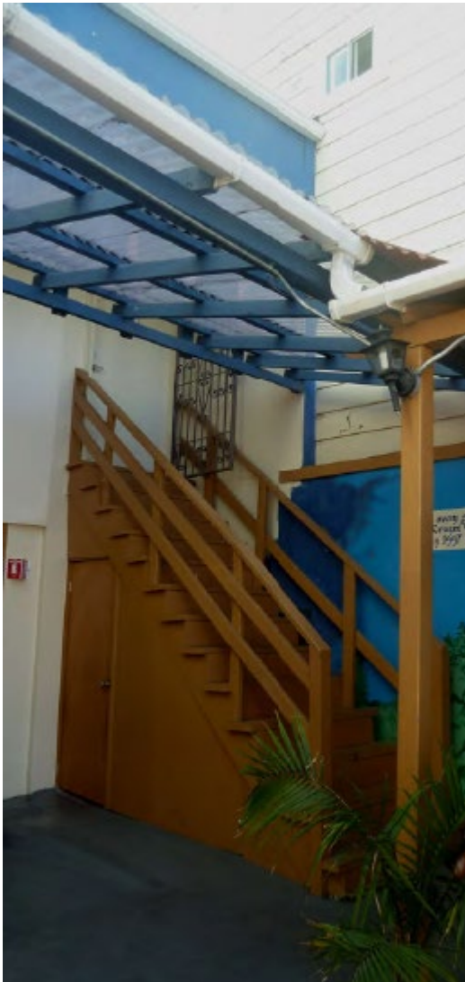
Casa Sanchez (2778 24 th Street Left: Sstairs at rear elevation, view southwest, 2016. Below: Ancillary building at rear of parcel, view north, 2016. Source: Casa Sanchez National Register Nomination
