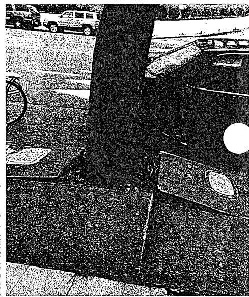
Sidewalk repair needs
