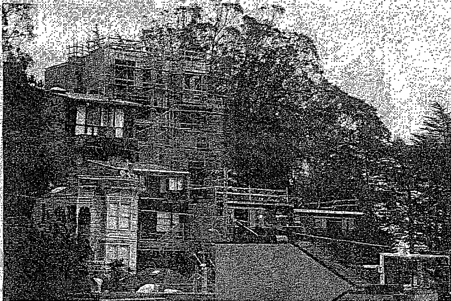
A six-story building is under construction on States Street amid Corona Heights' cottages, staircases and winding lanes. Lisa Sordahl / The Chronicle
