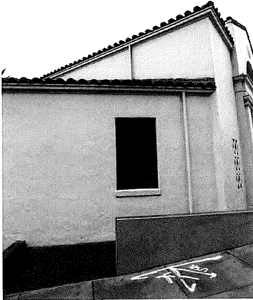
Figure 12 - The downspout from the upper roof sheds water onto this area of the lower roof, which bypasses the gutter and spills onto the ADA ramp into the Entry Pavilion. Photo by Page & Turnbull, 2017.
