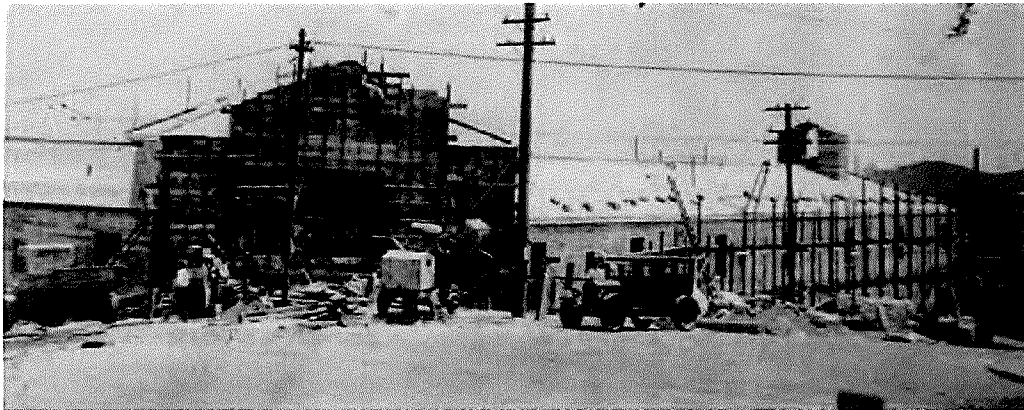
Figure 1 - Anderson (Woods) Hall under construction (ca. 1926). Source: San Francisco State University Archives
