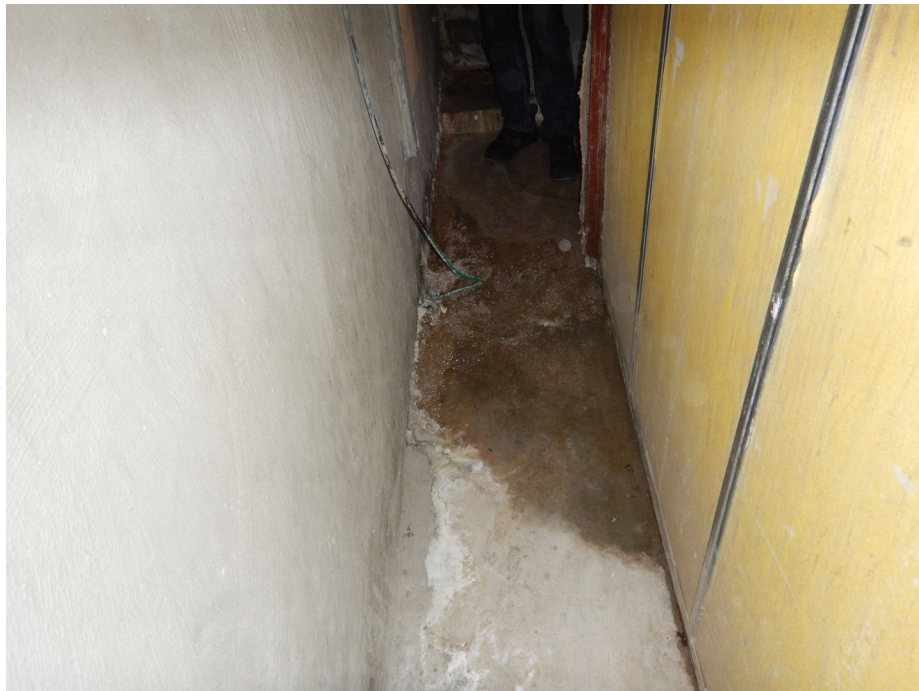
Photo 6: Efflorescence on wall base and water on floor adjacent to equipment (left side).
