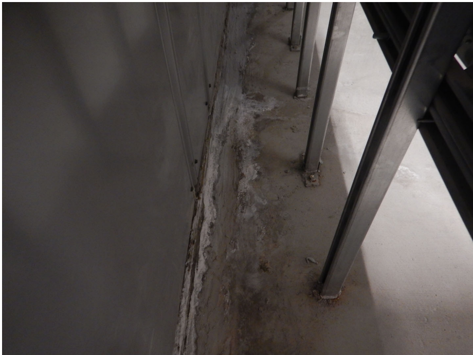
Photo 4: Efflorescence on side of concrete platform in middle of electrical room.
