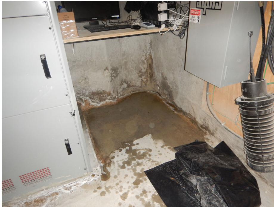
Photo 5: Efflorescence on wall base and water on floor adjacent to equipment (right side).
