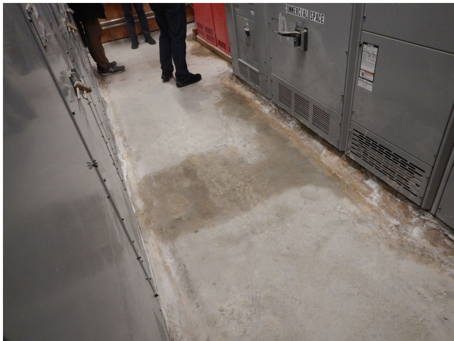
Photo 2: Efflorescence and water on floor in front of electrical equipment.
