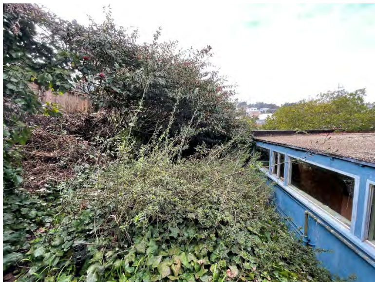
651 Duncan Street, rear elevation and overgrown yard, view west, 2020 Source: YA Studio
