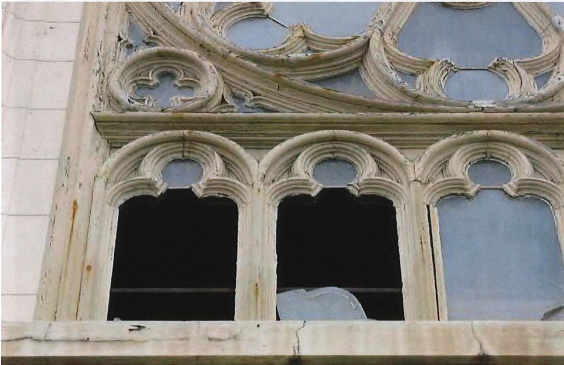
Figure 38c. West transept rose window, showing paint loss and missing glazing.
