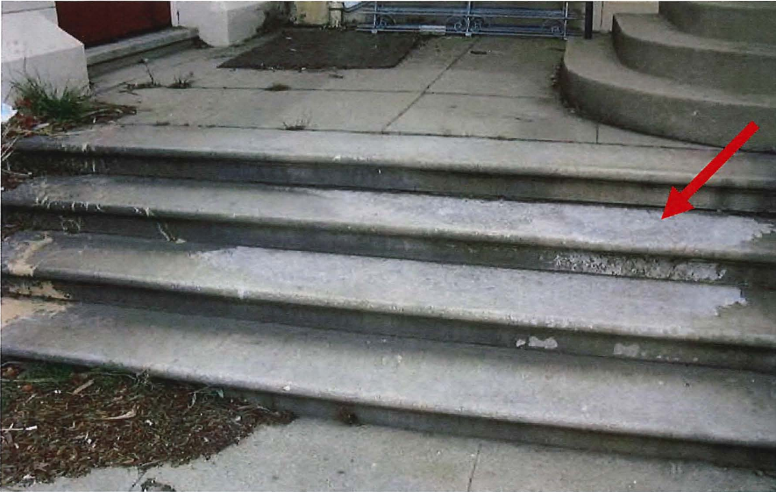
Figure 33d. West transept, south portal steps, showing paint stains (left), soiling and spalling surface (arrow).
