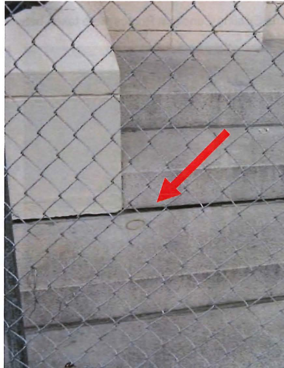
Figure 33b. Detail, east side of main portal steps, showing gap between blocks (arrow) due to uneven settling.
