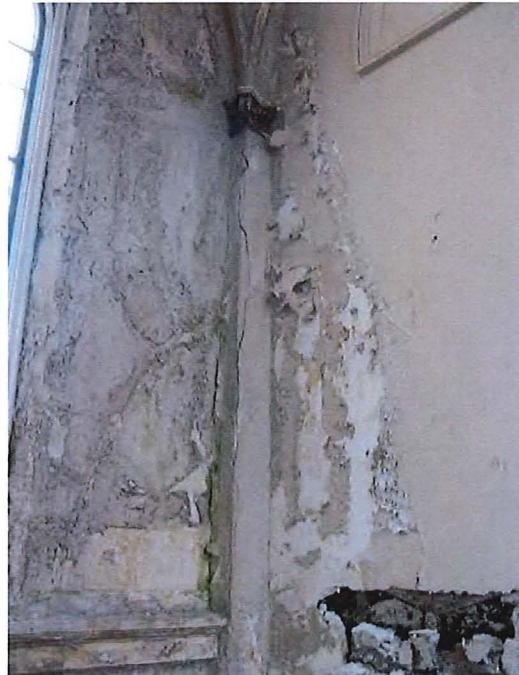
Figure 40d. Structural cracking and separation of plaster details from masonry substrate caused by moisture from blocked drains.
