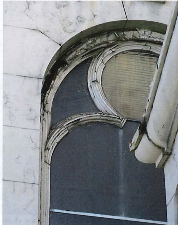
Figure 38b. East façade, transept window, showing soiling, paint loss and rotting/loss of tracery elements.
