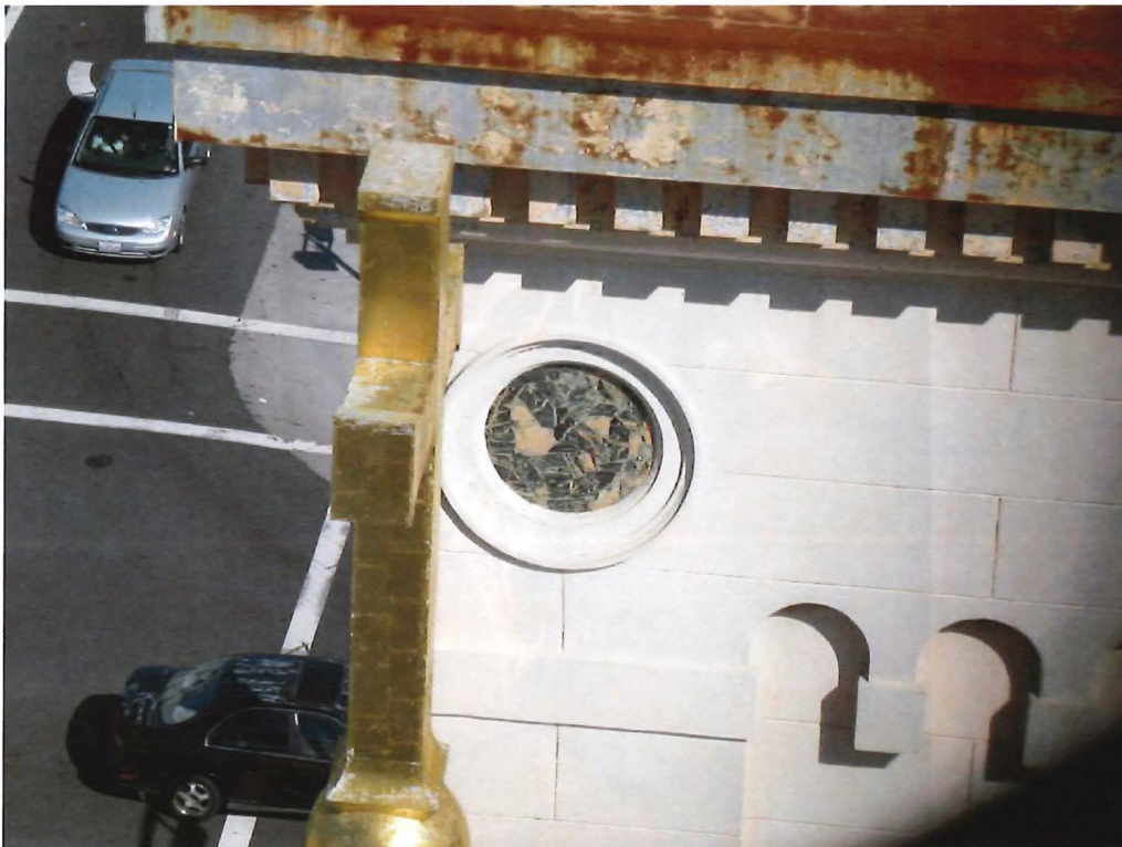
Figure 36b. The rooftop crosses require minor sheet metal and gilding repair.
