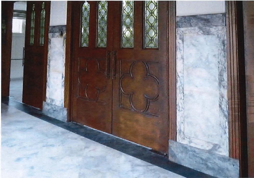
Figure 63. Marble wainscoting and interior doors of the narthex, after restoration (Page & Turnbull, 05/25/2018)
