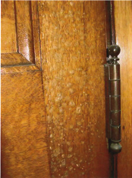
Figure 41a. Blistering of varnish on an oak door caused by moisture penetration.
