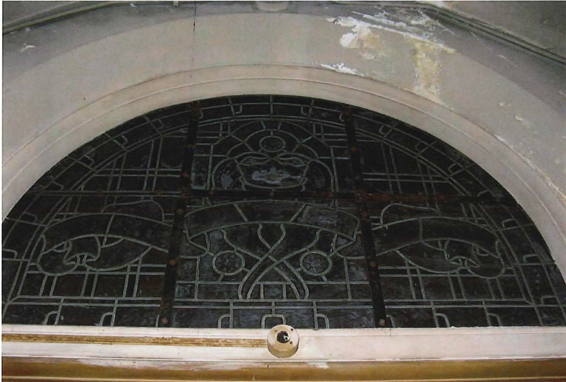
Figure 42a. North-east transept portal, showing blocked figurative stained glass window with heavy soiling and corrosion of steel frame
