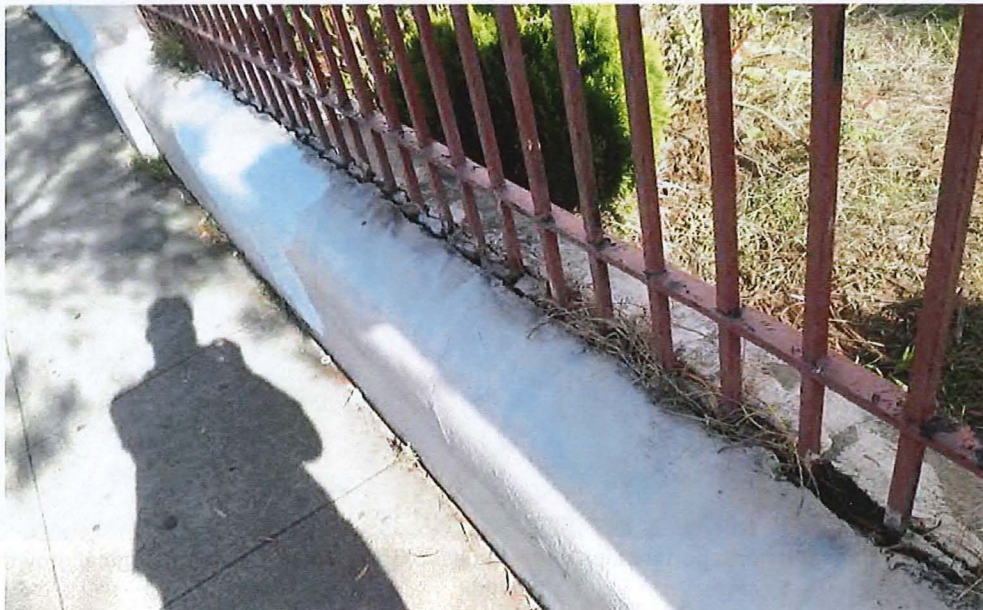
Figure 32c. Low brick wall along Howard Street, showing gaps and voids, corroded metal fence, and graffiti (painted over with mismatched paint).
