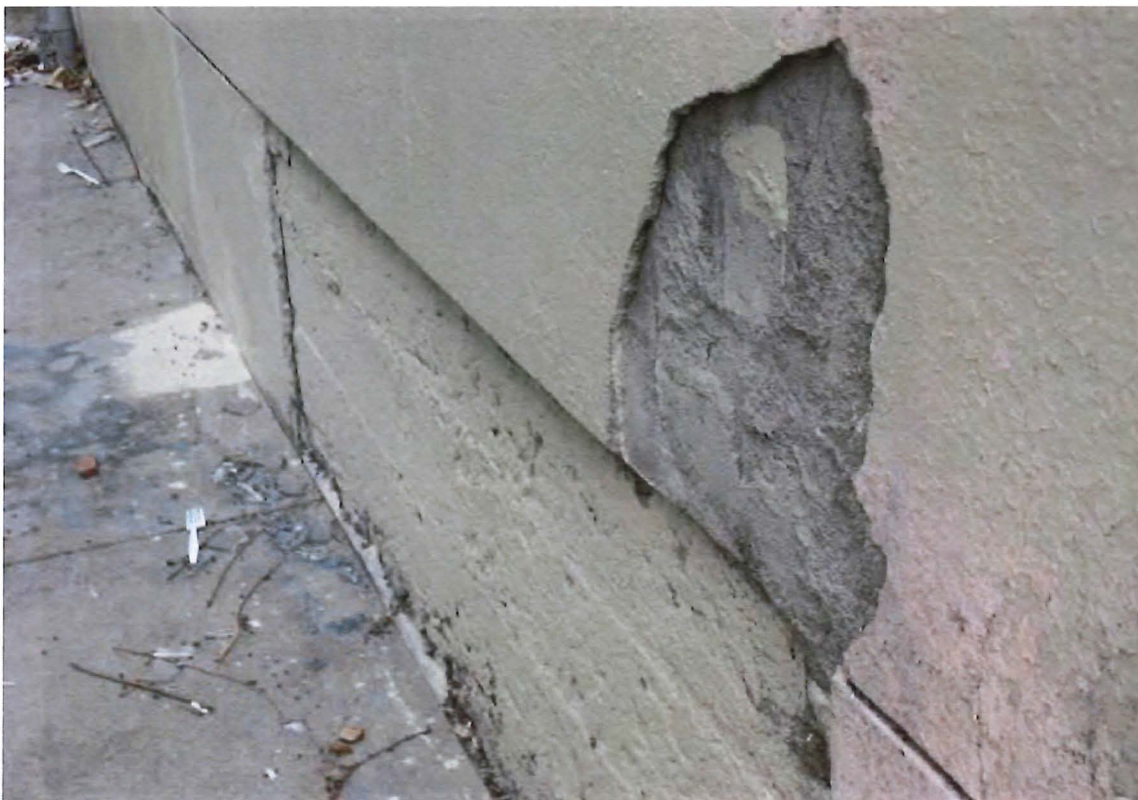
Figure 34b. East tower, north façade, showing loss of stucco at ground level.
