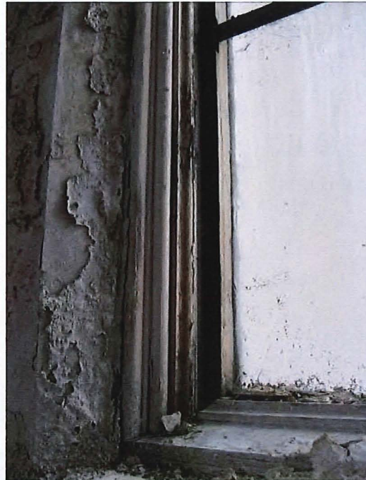
Figure 40b. Deterioration of plaster caused by moisture from poorly sealed window.
