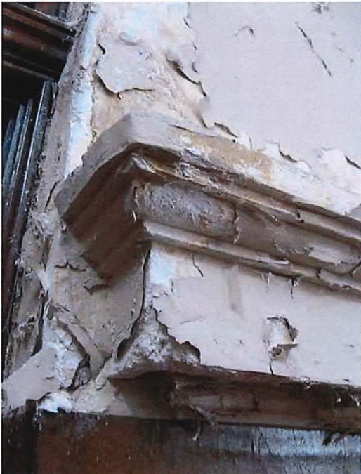
Figure 40c. Softening and deterioration of decorative plaster elements caused by moisture from faulty roofing.
