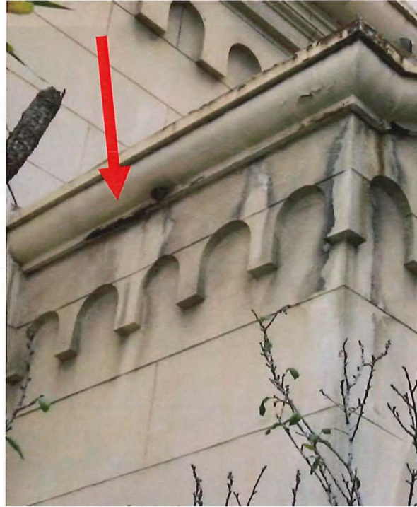
Figure 37b. Cornice above north portal, east transept, showing perforation (arrow) of the metal due to corrosion.
