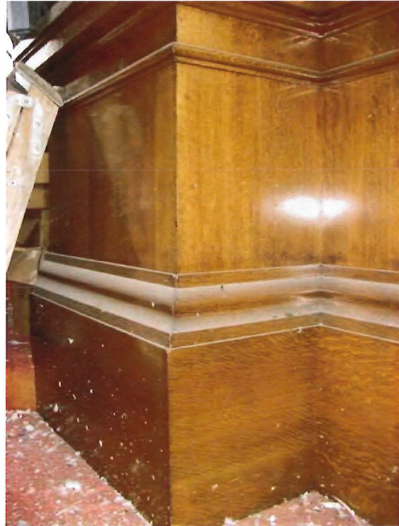
Figure 41b. Dust (on molding) and paint/guano spatters can cause permanent damage to wood finish.
