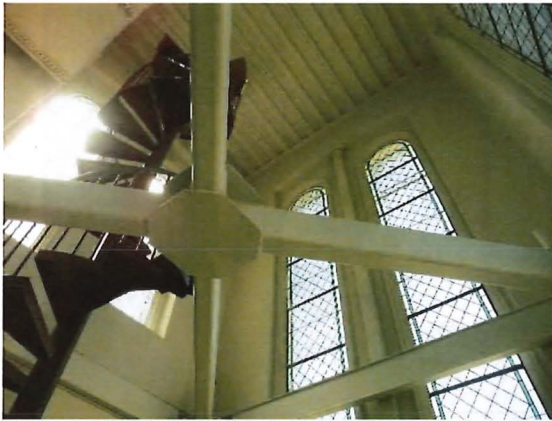
Figure 28. West tower, featuring seismic bracing and a spiral staircase. Source: Page & Turnbull, April 2019.
