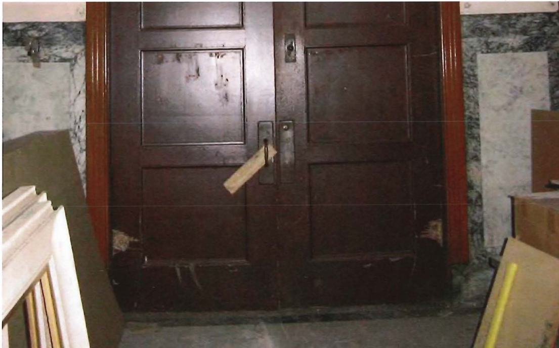
Figure 39a. Marble wainscoting of the narthex, showing soiling of the baseboard, wear of polished surface, and adhered tape. Original marble floor was covered with vinyl tile.
