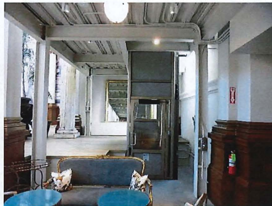
Figure 25. Wheelchair elevator accessing the mezzanine at the west end of the apse, looking south. Source: Page & Turnbull, April 2019.
