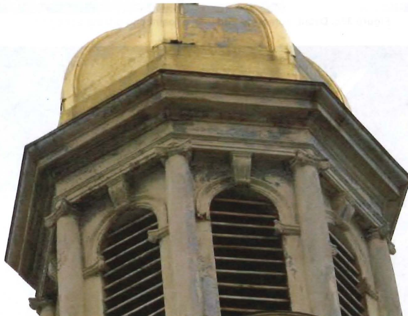
Figure 37c. East tower detail, constructed entirely of pressed sheet metal, showing missing architectural detail, loss of gilding and protective paint, and corrosion stains. Birds were nesting inside the towers.
