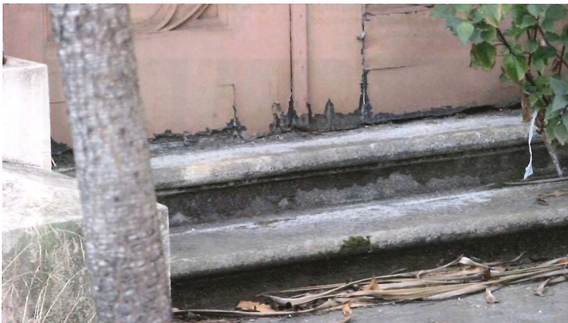
Figure 33c. East transept, north portal steps, showing decorative bull nose with biological growth and soiling.
