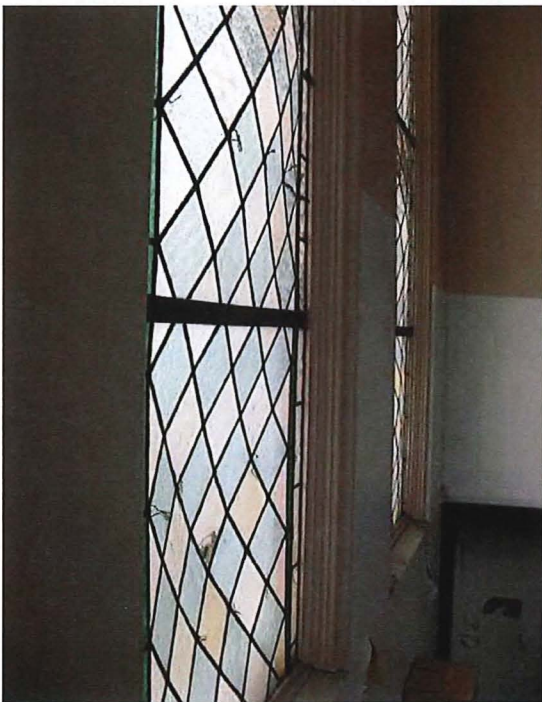
Figure 42 b. East tower, east windows, showing bowing of windows due to sagging lead comes or detachment from saddle bars.
