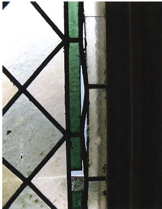
Figure 42c. Breakage and loss of colored glass panes due to distortion of lead comes.
