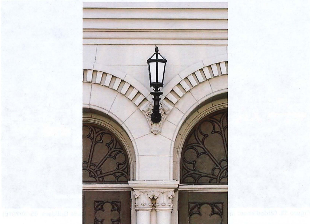
Figure 53. Exterior lighting fixture above main entrance on north façade (Rich Stapleton, 05/21/2018)
