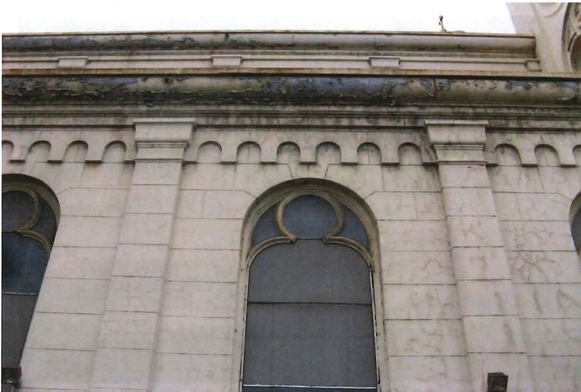
Figure 34a. East nave façade, showing soiling, water staining and hairline cracking of stucco.
