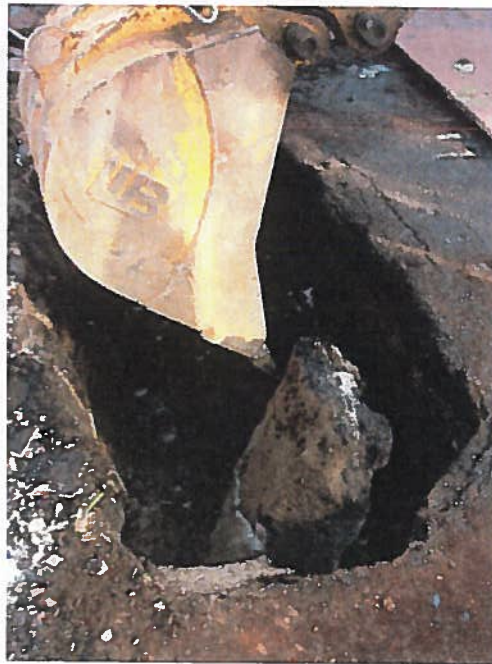
Photo 4. Excavation at broken storm drain pipe
