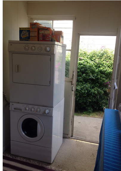
Back room - Laundry units
