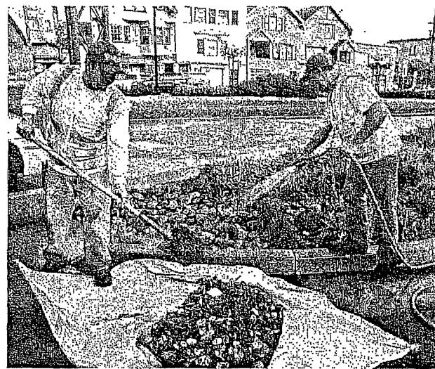
Maintenance workers remove sediment from a sediment basin in a bioretention planter on Cesar Chavez St in San Francisco. Photo: Robin Scheswohl
