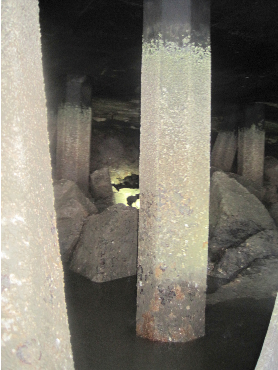
Photo 4. Undermining of seawall
