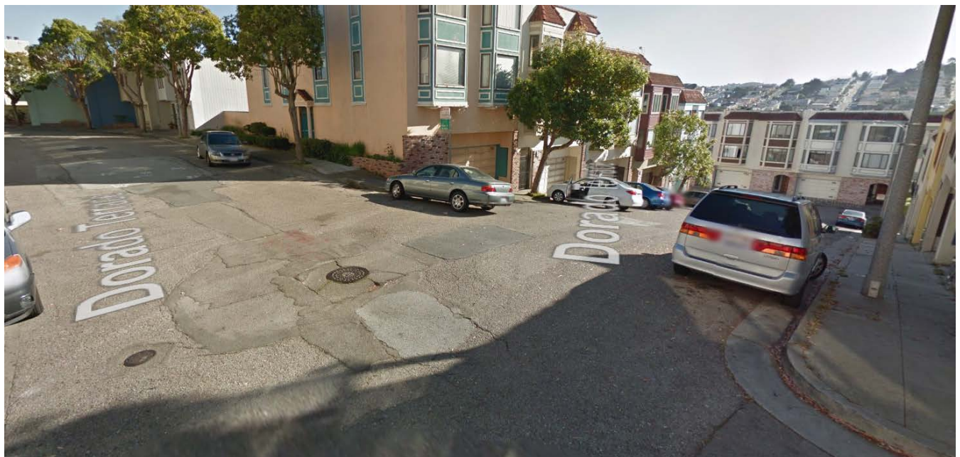
Figure 6: Condition of Project (Dorado Terrace)
