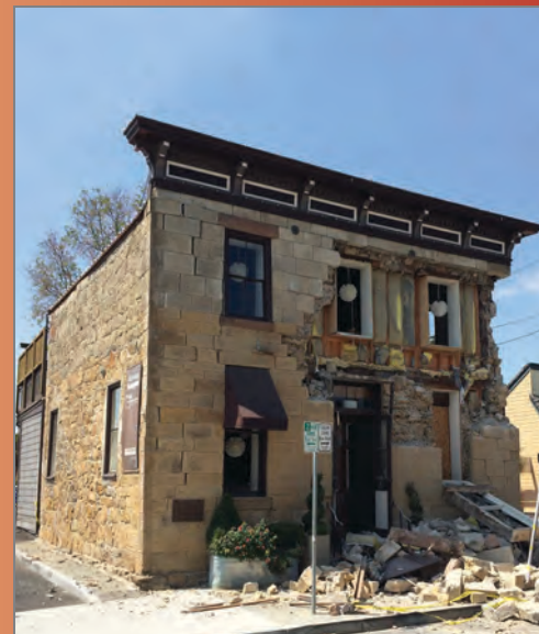
Damaged building in downtown Napa. Photograph by Erol Kalkan, U.S. Geological Survey.
