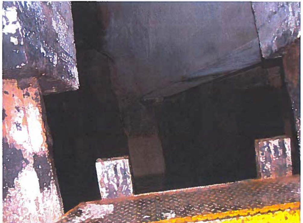
Figure 27 - Sunken Slab on Pier 31.5 (5/15/19)
