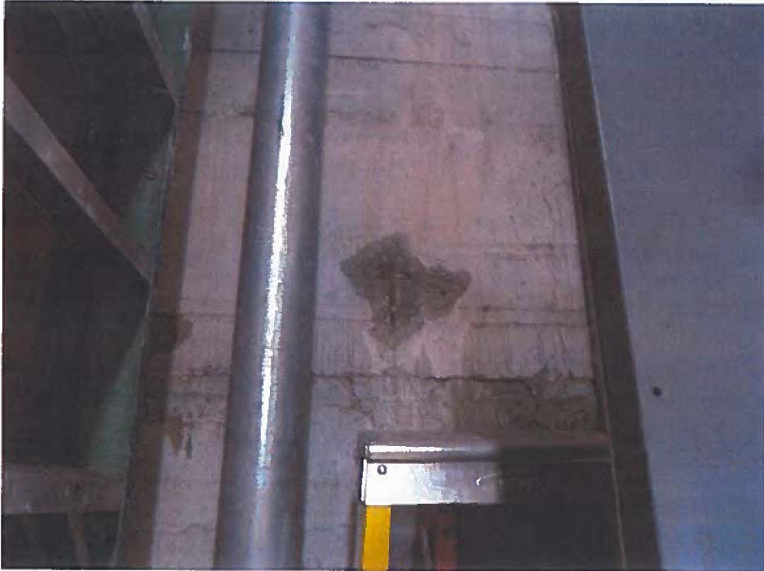
Figure 14 - Spalling at interior face of concrete wall
