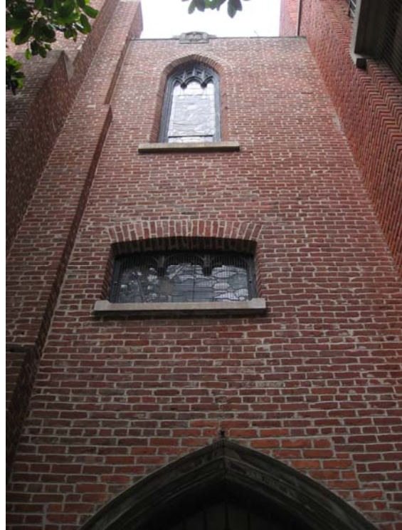
Closer view of upper two stories of west bridge connector. (Page & Turnbull, March 2013)
