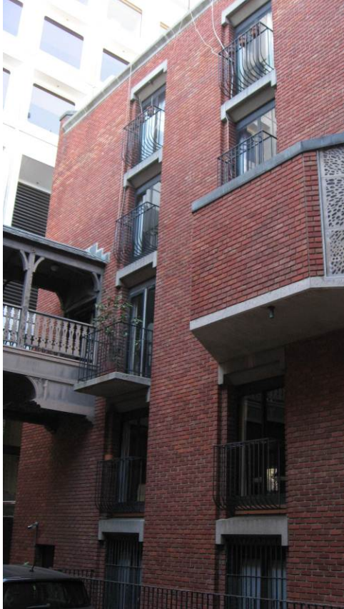
Detail of the east end of the rear (north) façade, looking southeast. (Page & Turnbull, April 2013)
