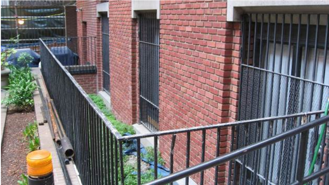
Detail of ground floor window well along rear (north) façade, looking southeast. (Page & Turnbull, April 2013)
