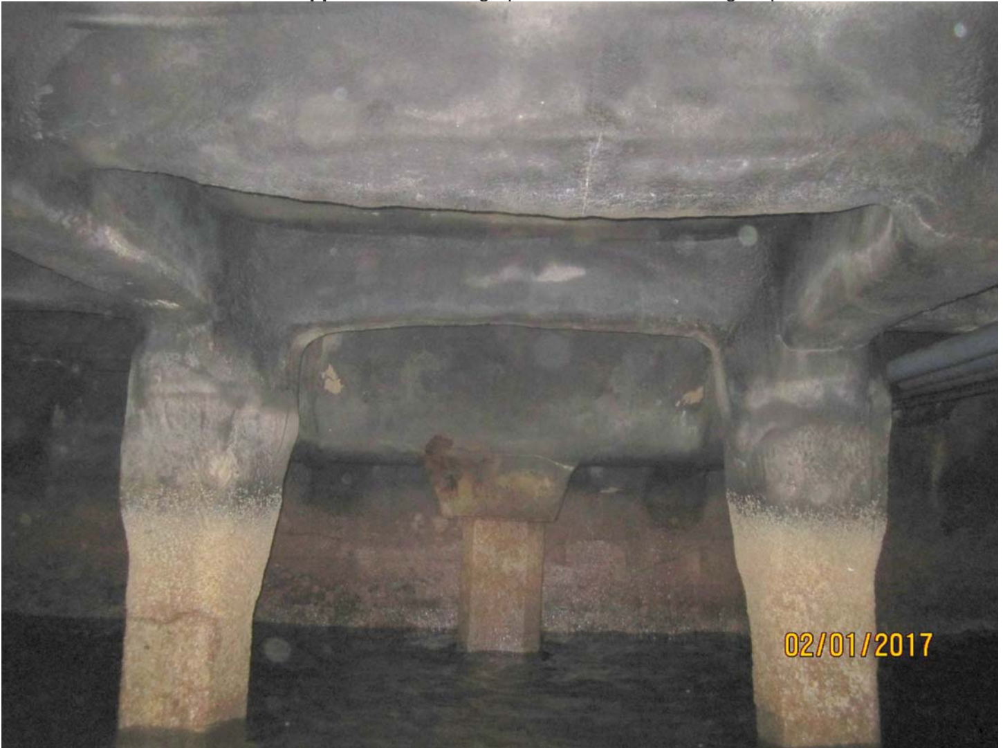
Photo 2. Typical condition of sea wall adjacent to Pier 9. No significant damage noted.
