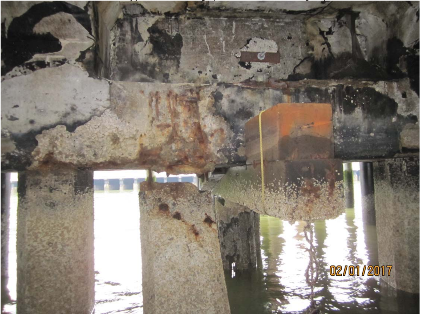
Photo 10. Conditions inside northern edge of pier. Many batter piles are broken in the north-east quadrant of the pier. Broken batter piles do not affect gravity load capacity of pier.
