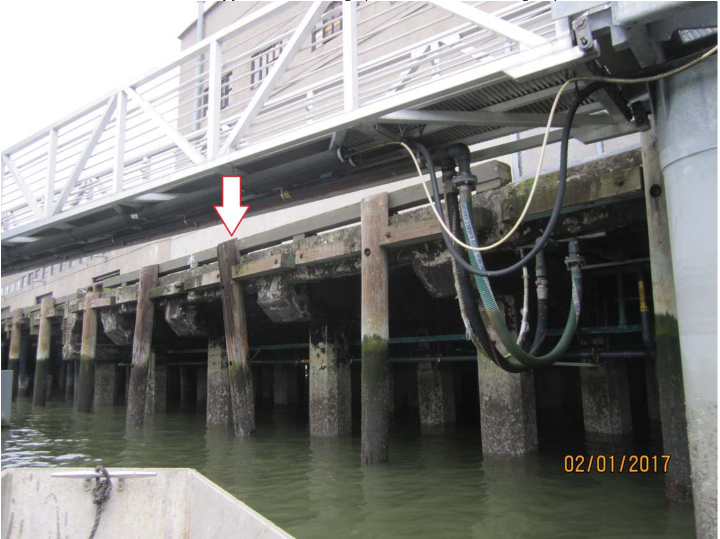
Photo 9. One broken fender pile on northern edge of pier near bulkhead building.
