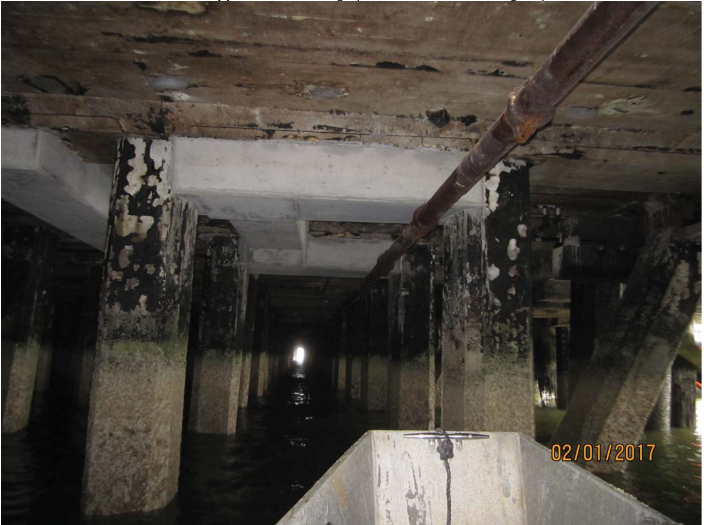
Photo 13. New concrete beams added along near south edge of pier. Could not locate drawings for this work.
