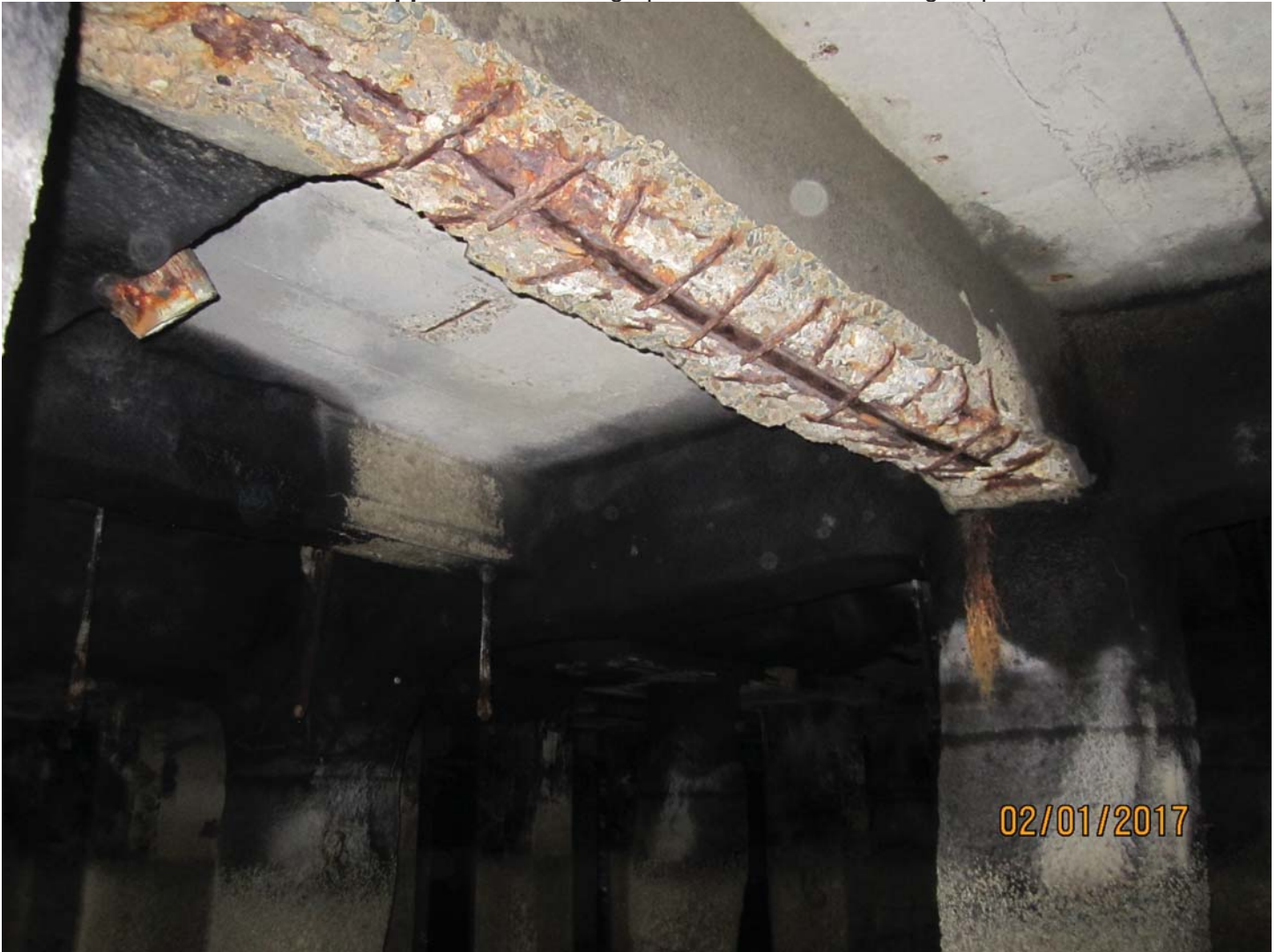
Photo 6. One concrete beam noted with severe spalling. Does not appear to have ever been repaired with shotcrete.
