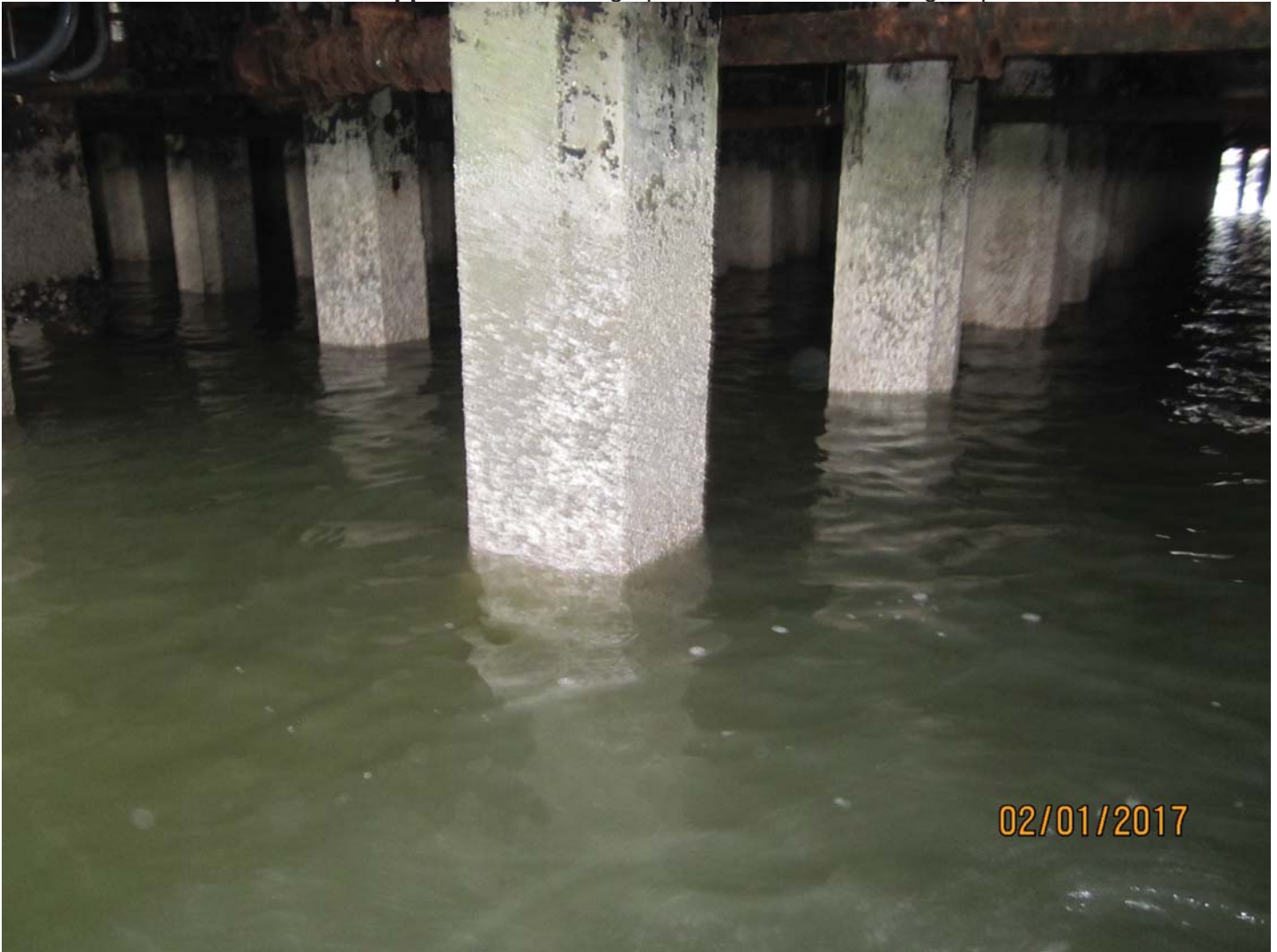
Photo 7. Minimal section loss at the concrete pile jackets near the waterline
