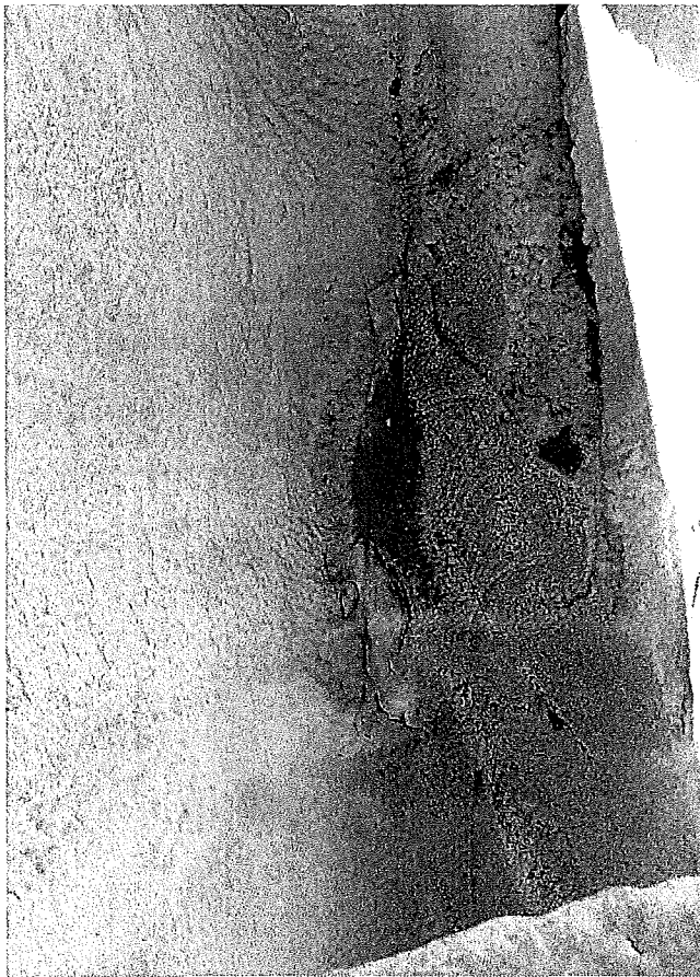
Figure 4. Detail of roofing membrane and localized damage; assess conditions throughout.
