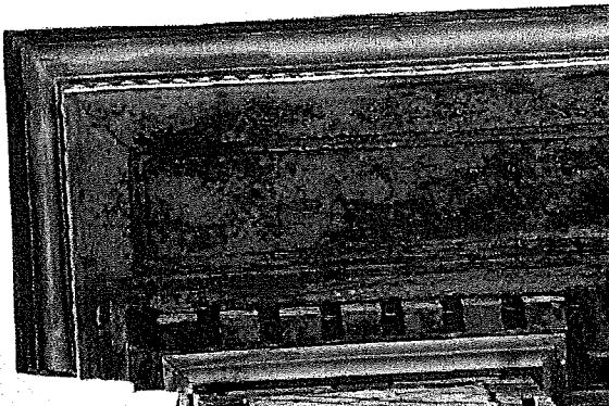
Figure 3. Cornice at northwest corner; localized areas of severe damage observed & requiring immediate repair.
