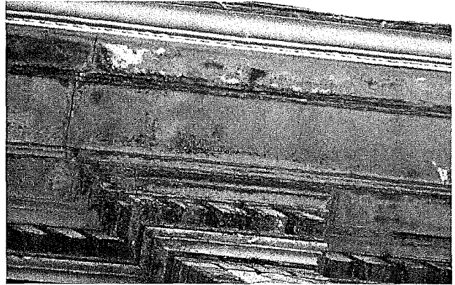
Figure 4. Cornice; conditions noted as typical.
