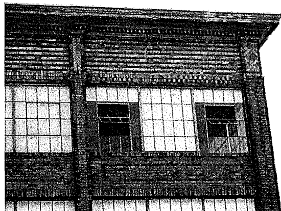
Detail of piers and cornice on the west façade. (Page & Turnbull, April 2013)
