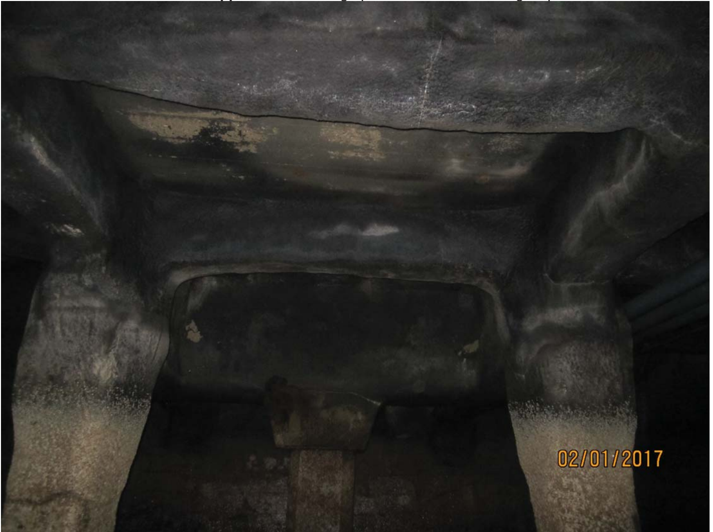
Photo 3. Typical conditions of marginal wharf under bulkhead building. Previous shotcrete repair in serviceable condition, some hairline cracks and scour.
