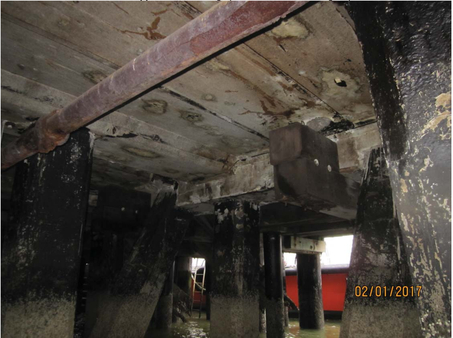
Photo 14. Typical conditions along southern edge of pier.
