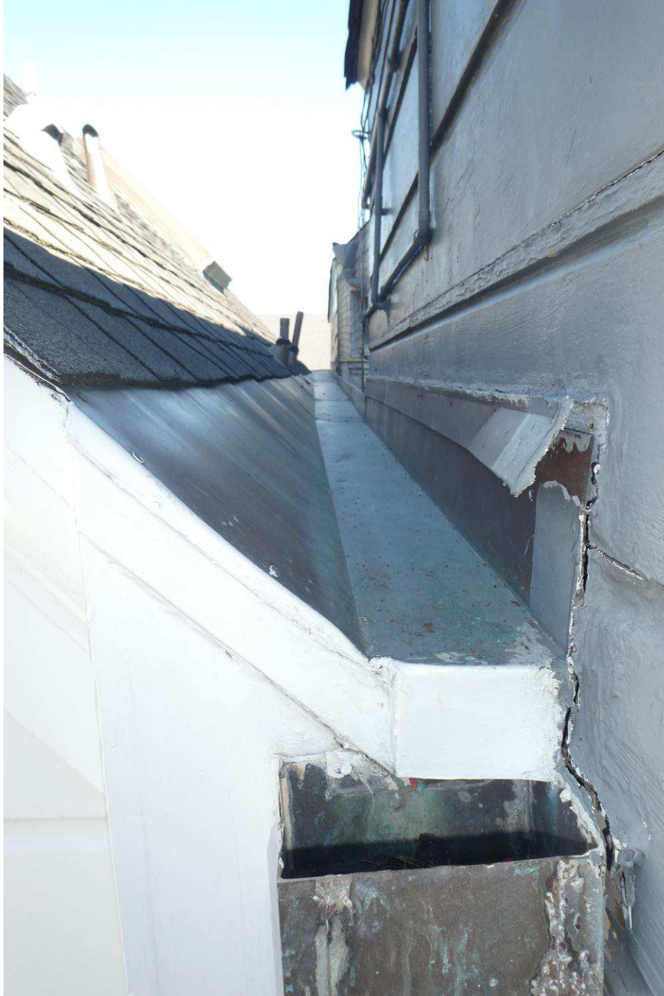
Figure 51: Copper gutter, counterflashing, and leader head where the main roof meets the neighboring building to the northeast.
