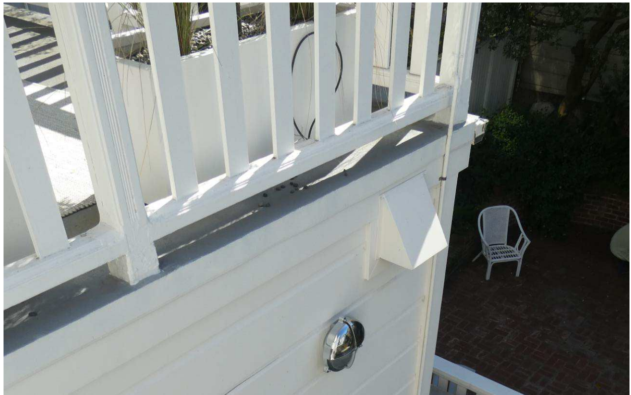
Figure 55: Detail showing the asphaltic roof at the decking above the first floor kitchen.
