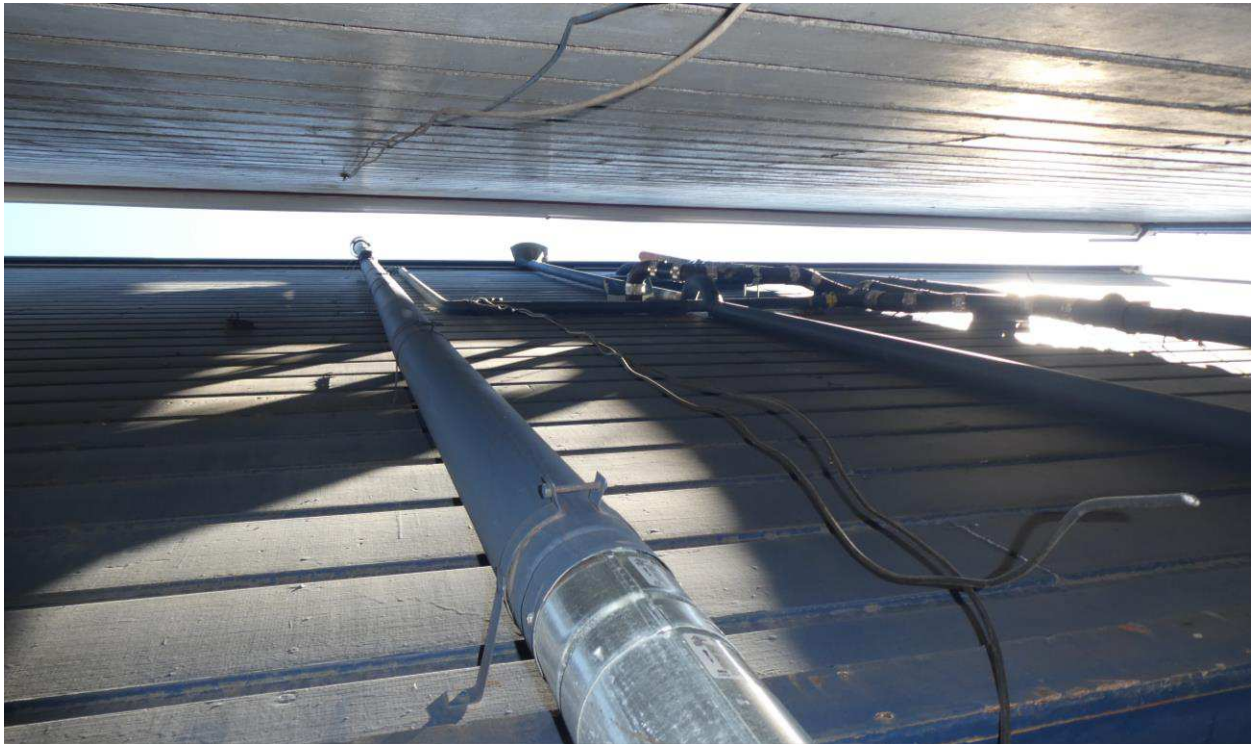
Figure 48: Detail showing the mechanical and plumbing flues/piping/conduits at the upper southwest wall.
