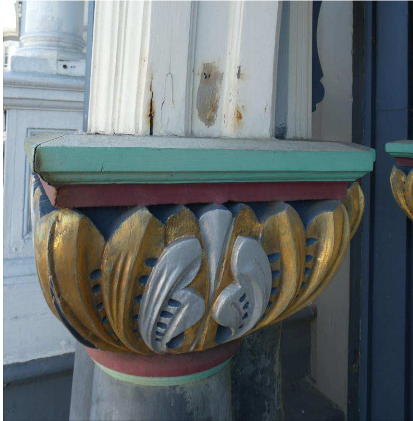
Figure 25: Detail of wood deterioration and checking/splitting at the main entry.
