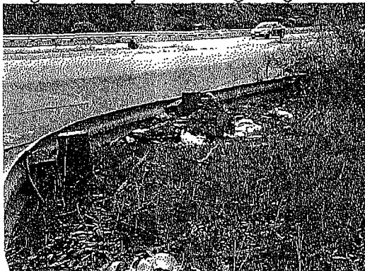
A typical trash site, dumped daily on Mansell St and other locations. The bags get torn open by animals and loose trash spreads to hillsides and meadows. Regular daily or weekly pick ups of these dump sites is not happening.
