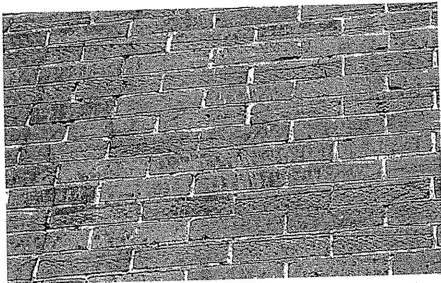
Detail of "scars" left by abrasive cleaning.
