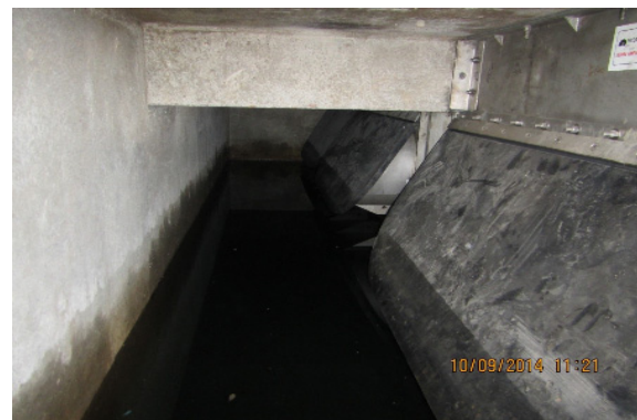
Typical backflow preventer device installed over the weir
