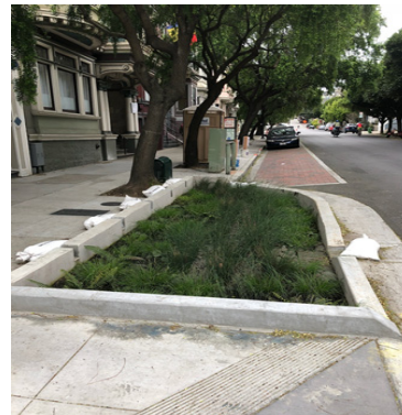
Completed rain garden and permeable paving parking strips at Waller and Steiner Streets
