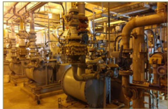
Oceanside Building 800 existing digester and natural gas compressors to be replaced as part of this project.
