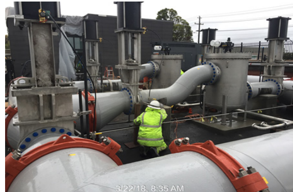
SEP 920 W3 Water Piping, Strainers and Knife Gate Valves
