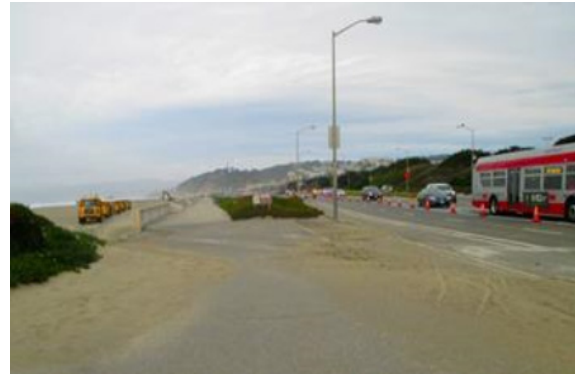
Contractor excavator and dump trucks loaded with surplus sand collected at North Ocean Beach
