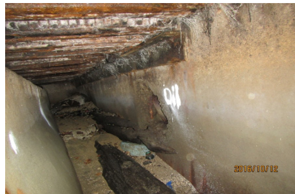
Beach St. CSD: Sewer structural corrosion and other deficiencies
