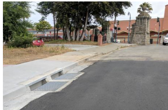
The project includes constructing new inlets to improve surface drainage in the Victoria/Urbano neighborhood
