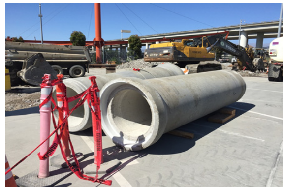
Preparation for Replacement of the Existing Sewer with New Reinforced Concrete Pipe
