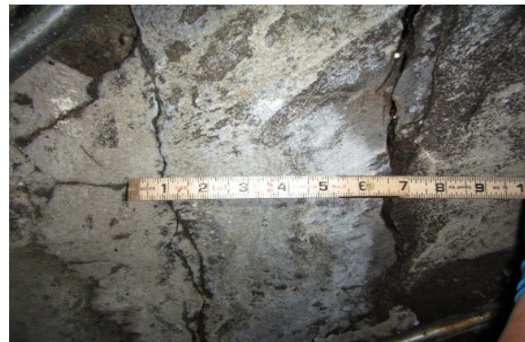
Extensive structural cracks at 5th St CSD
