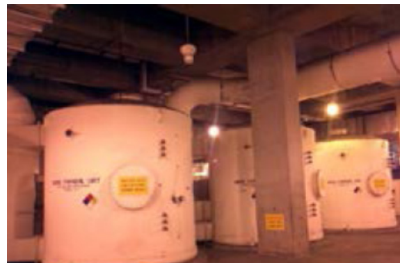
Existing OSP Odor Control Unit carbon media vessels
