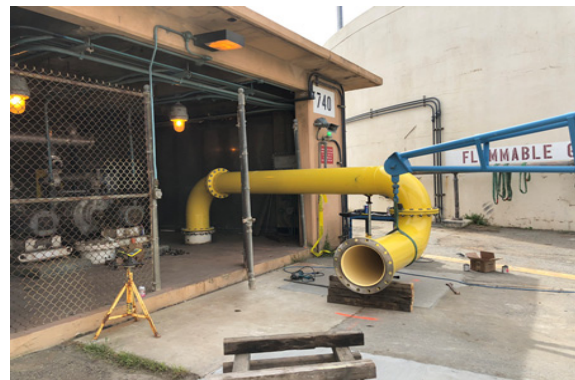
Installation of 18" Waste Gas Piping from Gas Booster Station (SEP 740) to Waste Gas Burners (SEP 821)
