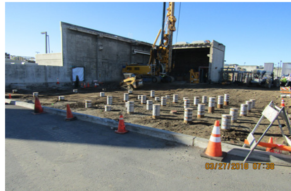
Completed Torque Down Piles and remainder of the Cryogenic Building SEP 270 shown
