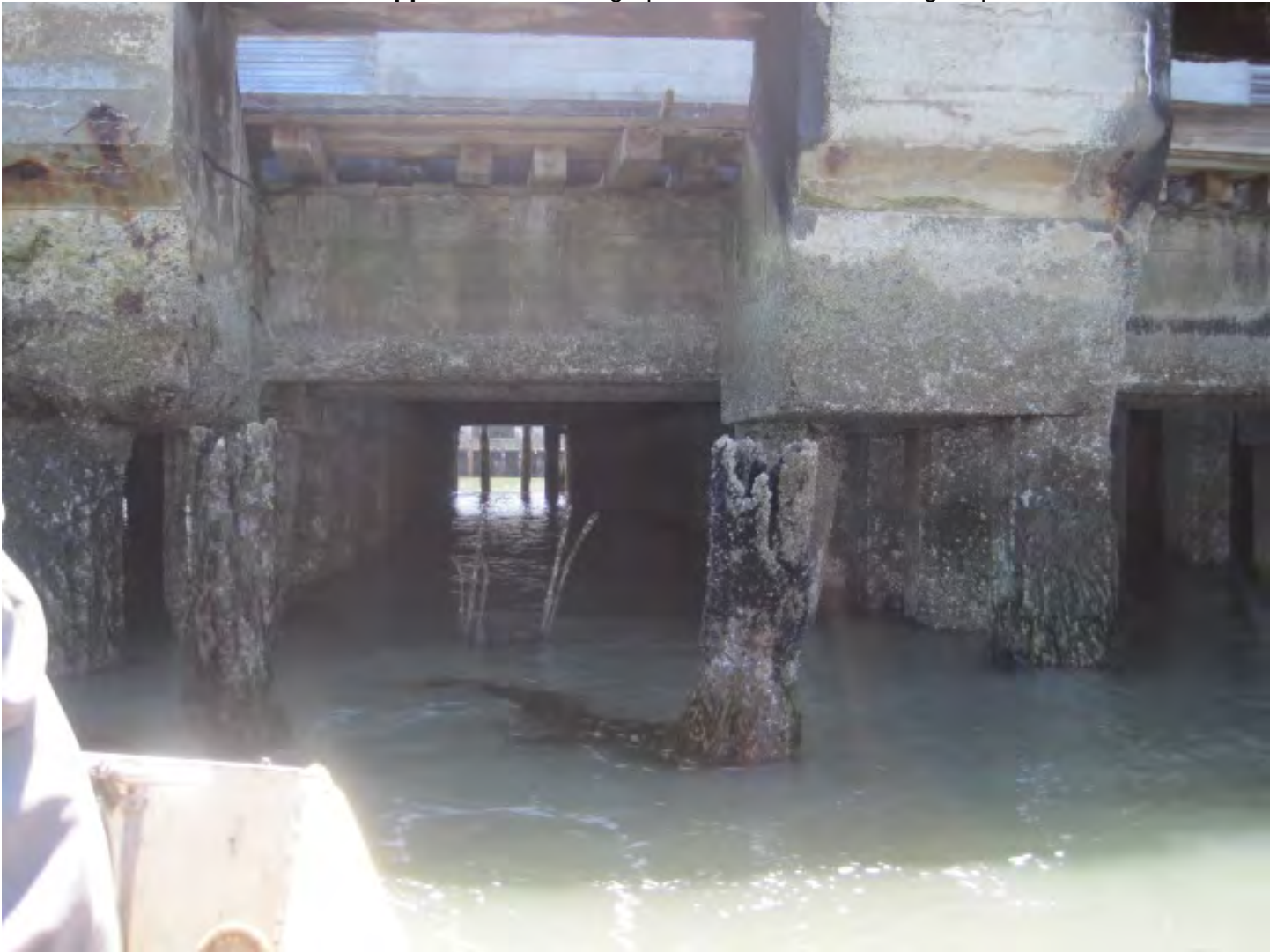
Photo 5. Deteriorated fender piles
