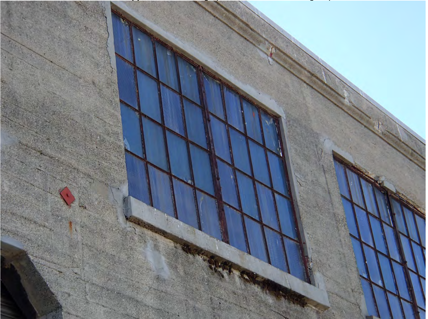
Photo 2. View of the concrete spalling at window openings at east elevation
