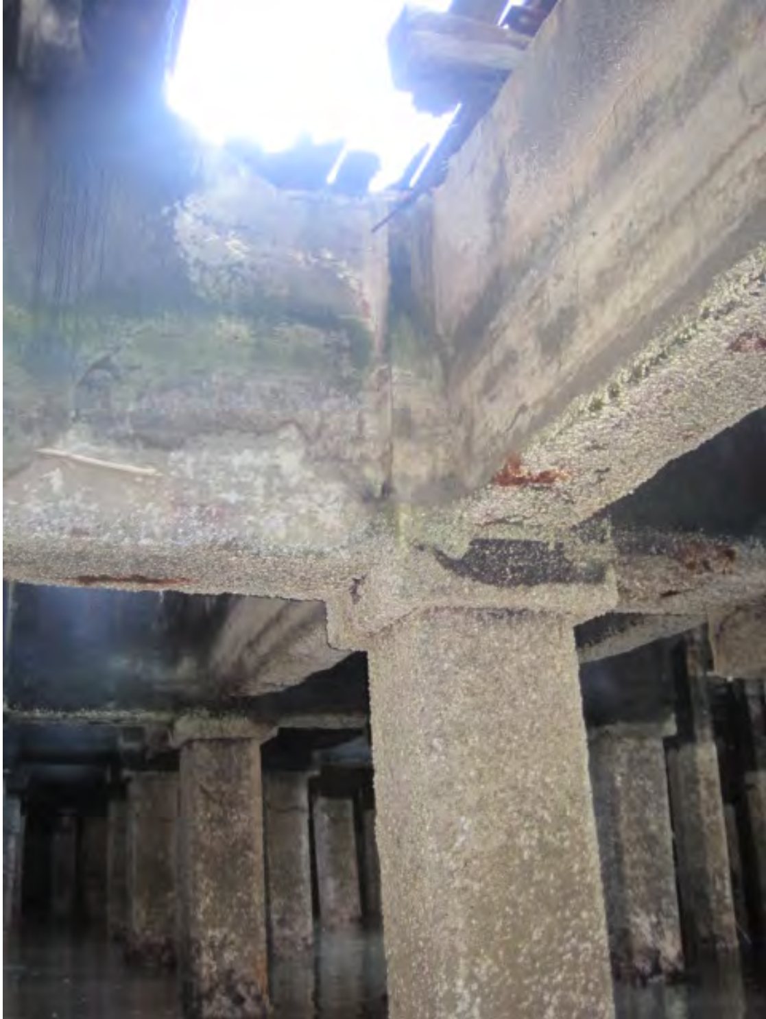
Photo 4. Hole at deck
