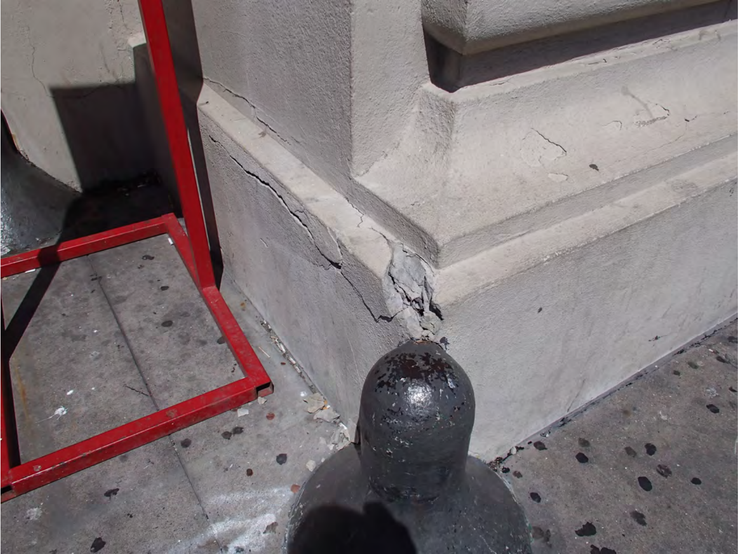
Photo 10. View of the stucco spalling in the wall base near the entrance
