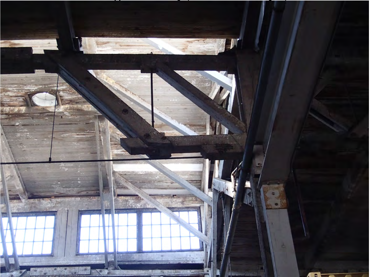
Photo 13. View of a modified timber roof truss. Note the water staining in the roof sheathing beyond
