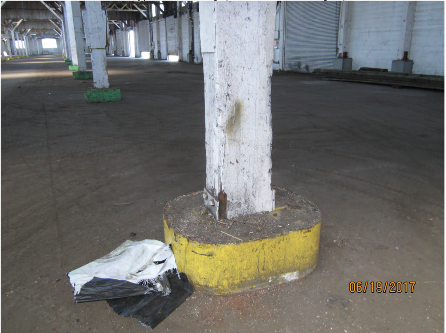
Photo 15. Interior wood columns on raised footings. Less susceptible to dry rot, but some have minor damage from vehicle impact.
