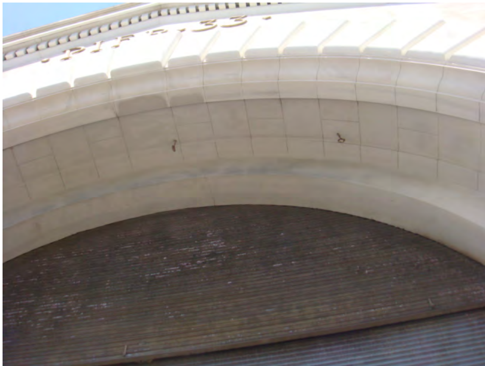
Photo 2. Rusting eye bolts
