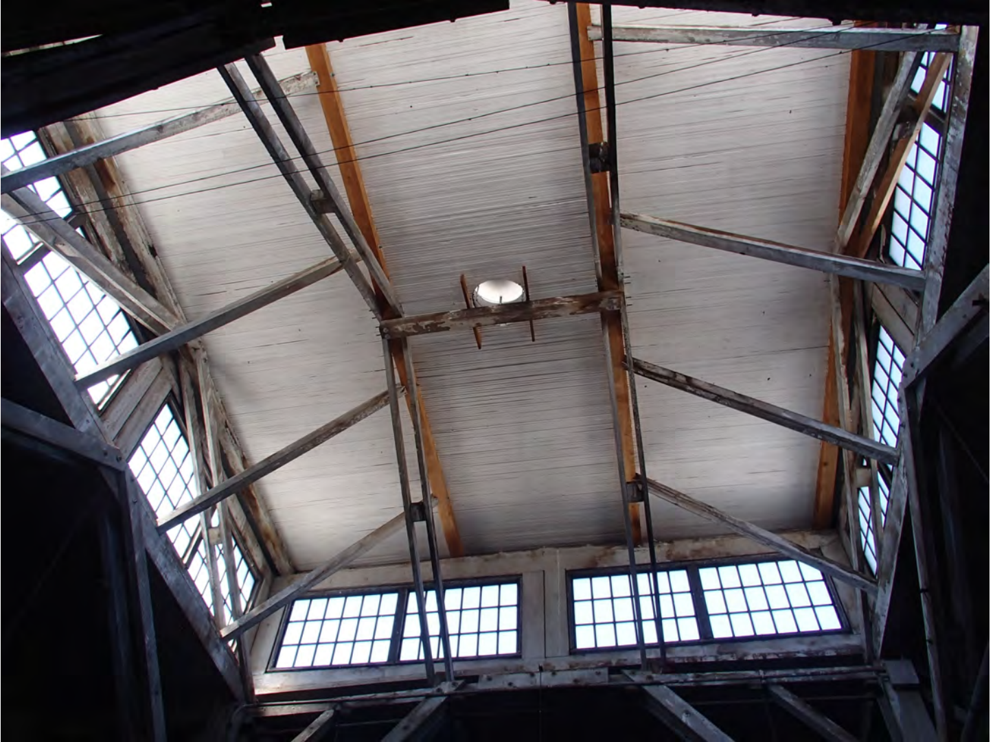
Photo 8. View of a timber roof pop-up area with shoring work on wood beams and replaced roof sheathing
