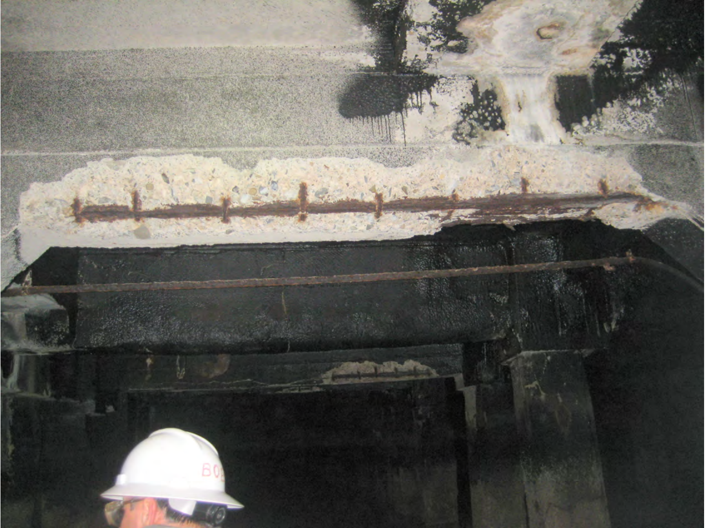
Photo 7. Spalling and exposed/corroded rebar at beam
