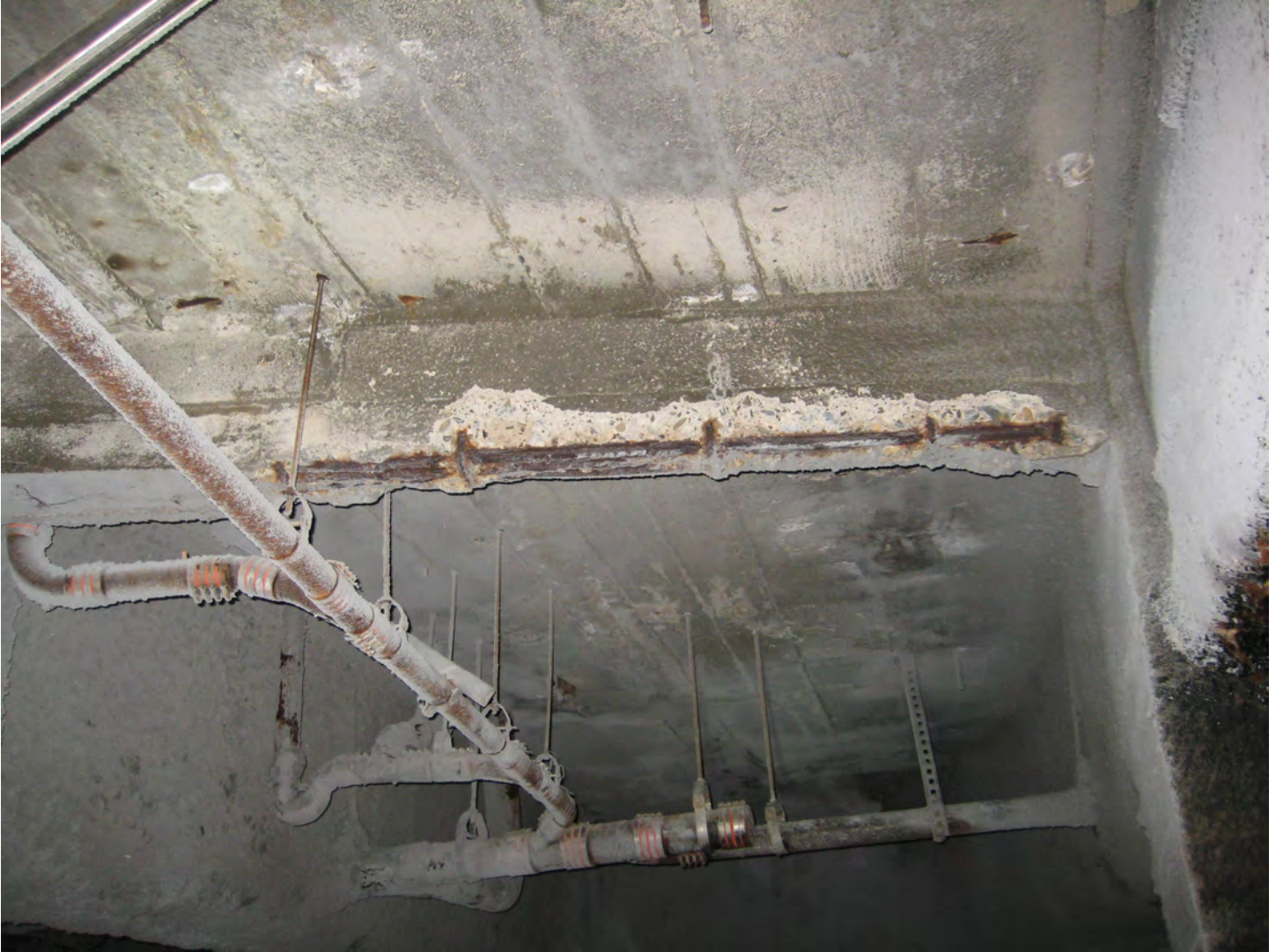
Photo 6. Spalling and exposed/corroded rebar on beam
