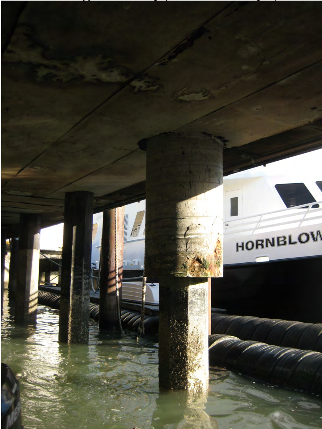
Photo 3. Crack on pile cap
