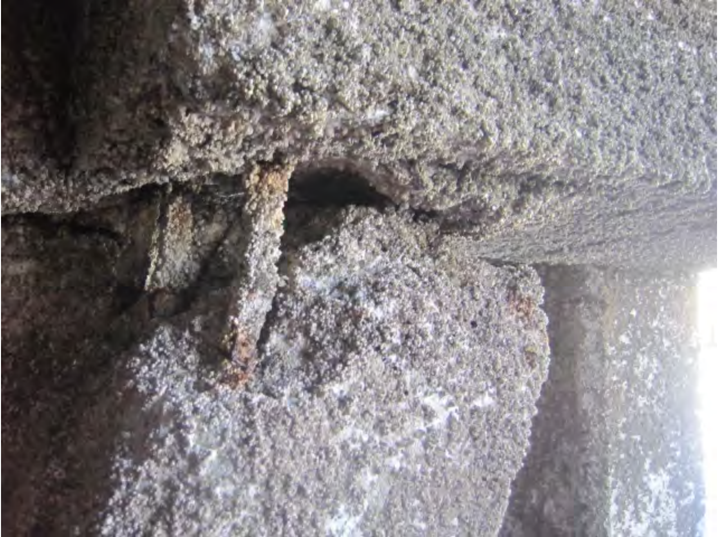
Photo 11. Close up of broken batter pile
