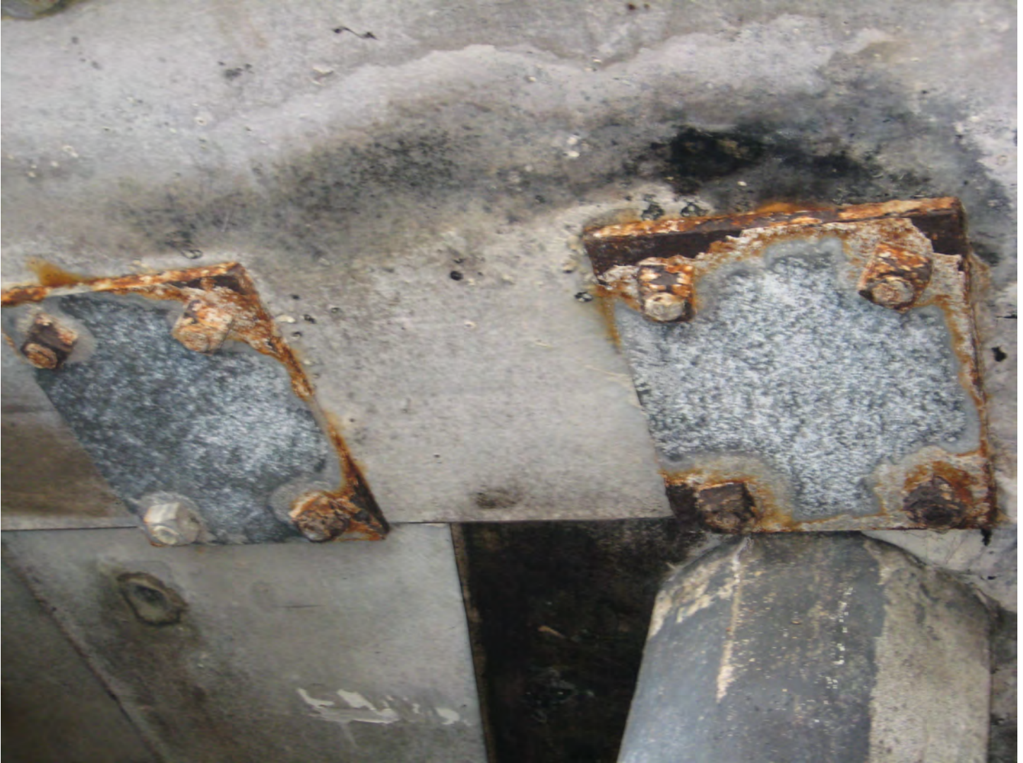
Photo 7. Corrosion on steel plates
