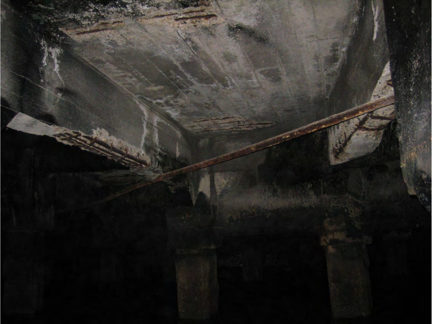
Photo 5. Spalling and exposed/corroded rebar on beams and slab
