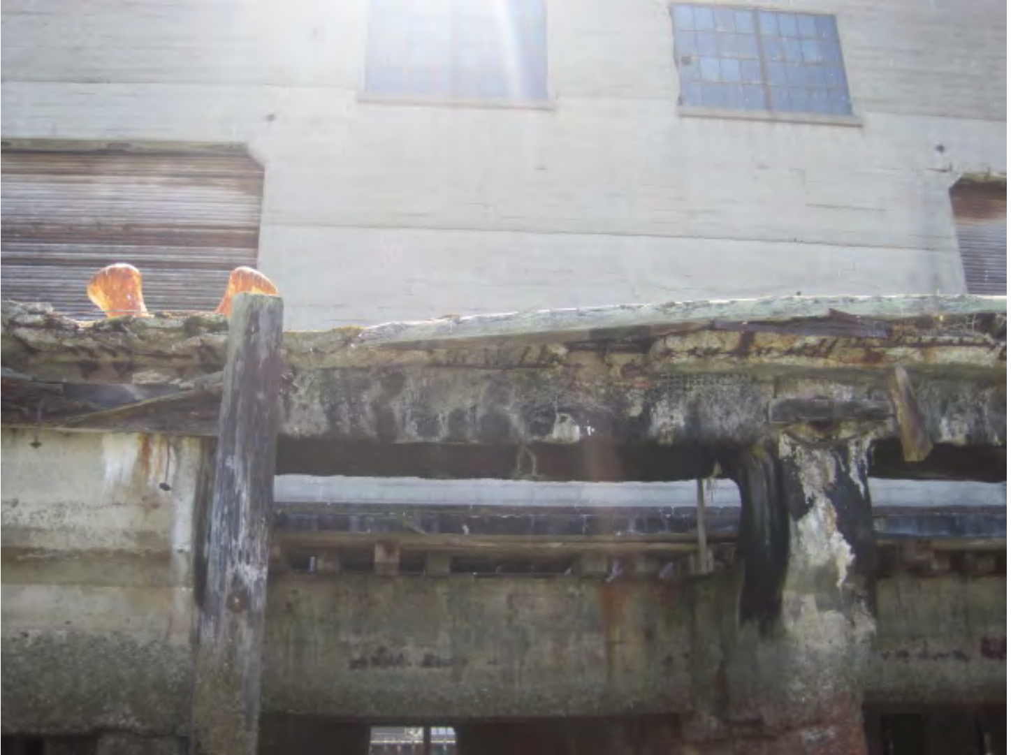
Photo 10. Spalling deck and corroded/exposed rebar
