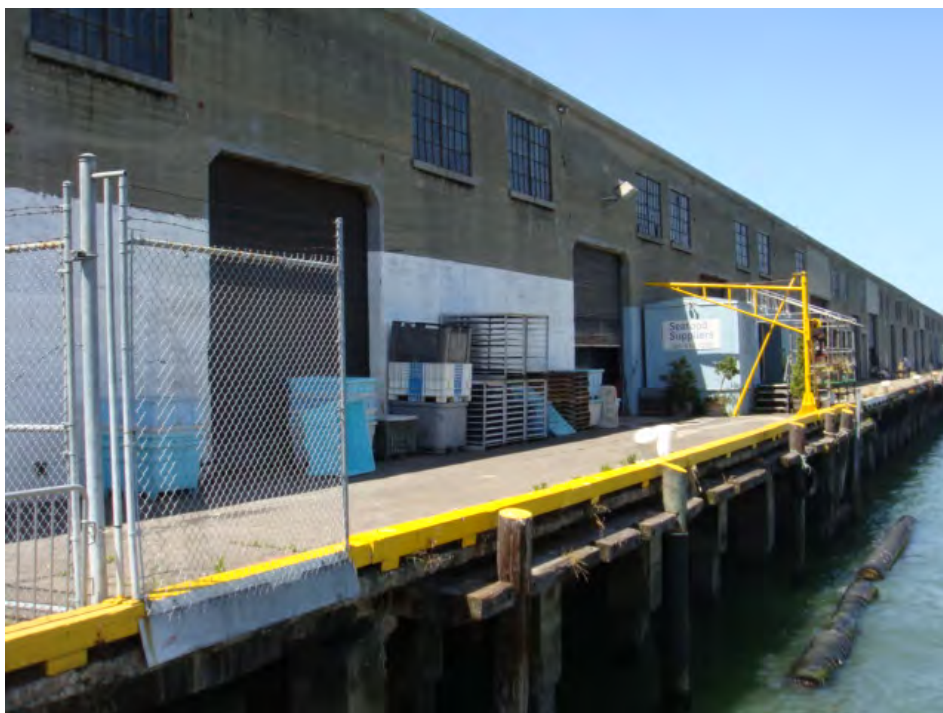
Photo 4. Concrete spalling around windows at east wall
