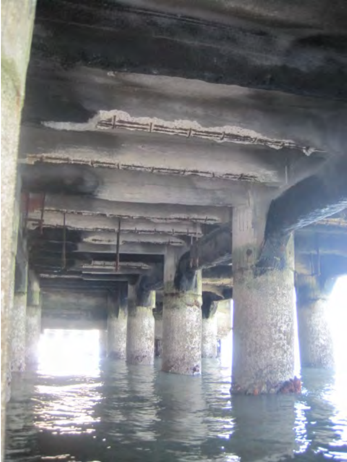
Photo 5. Spalling of concrete beam with exposed/corroded rebar
