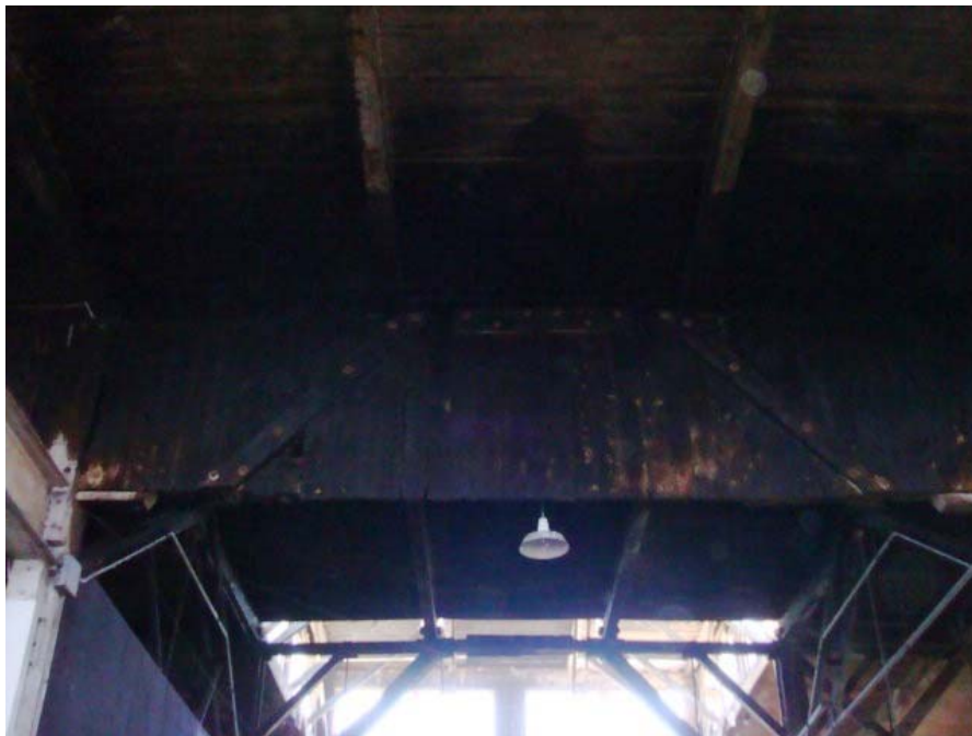
Photo 6. Fire damage at north end
