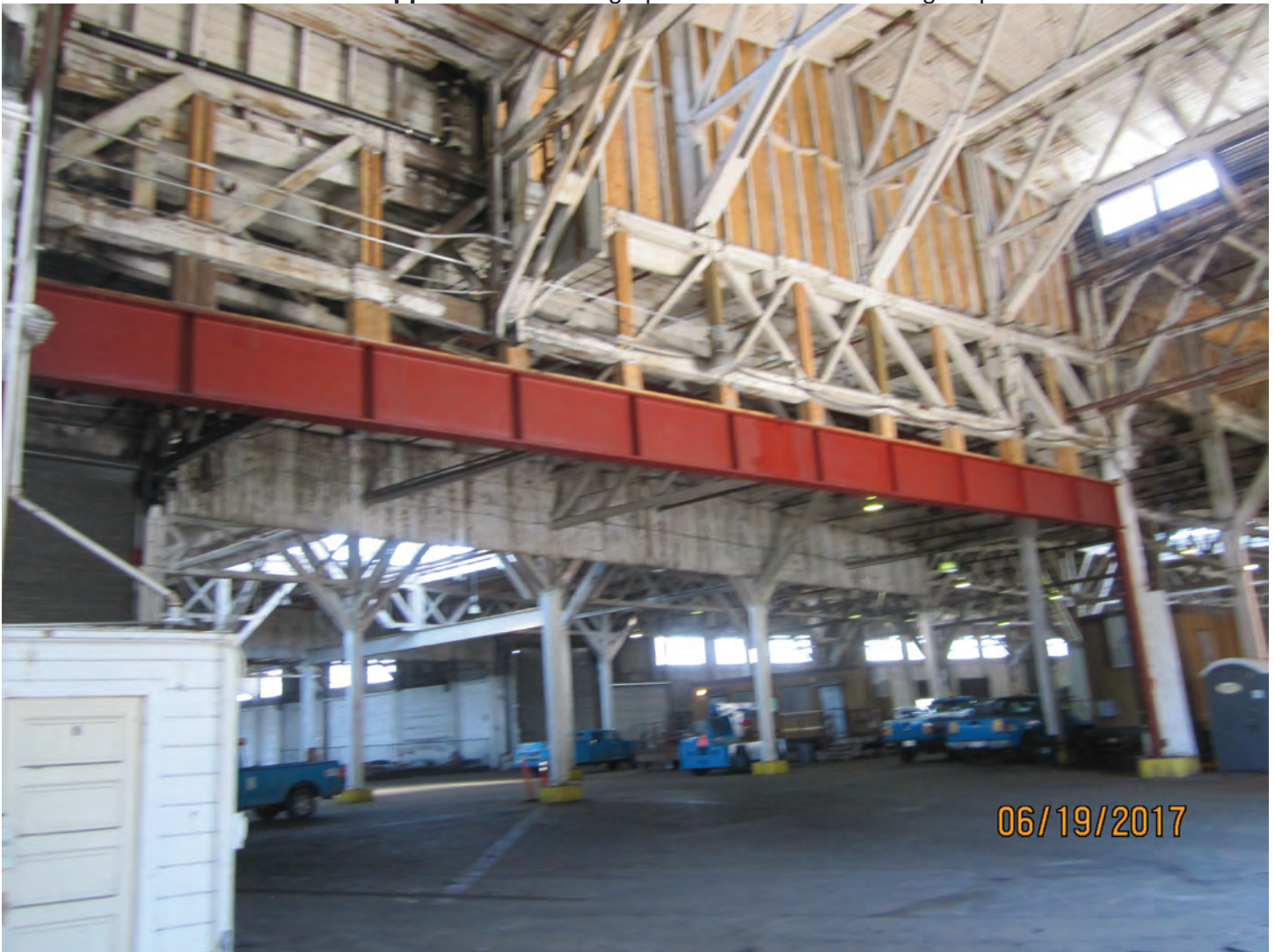
Photo 7. New steel beam and tube steel posts added in 2017 to strengthen existing wood truss.
