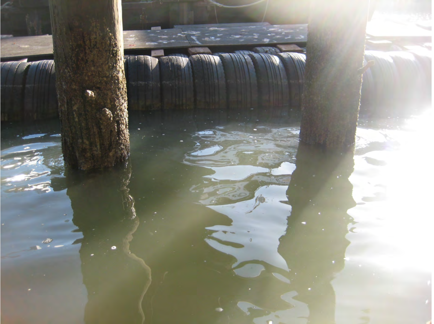
Photo 4. Deteriorated wood piles near metal deck
