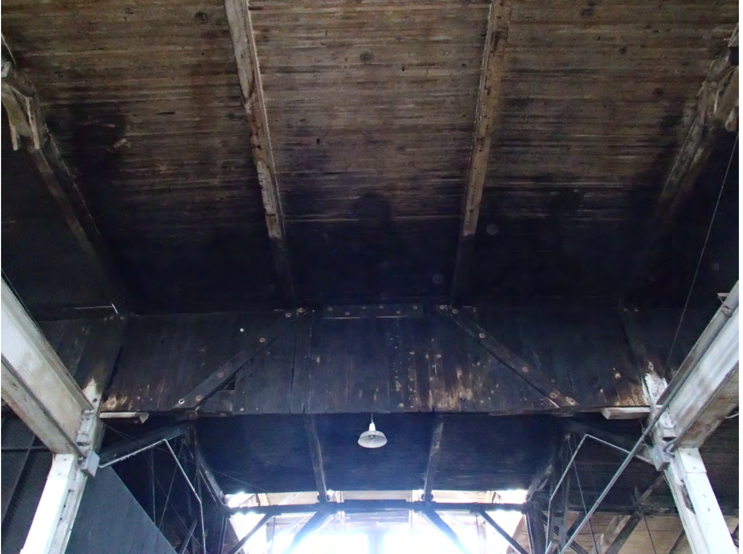
Photo 4. View of a portion of the roof displaying fire damage at the north end of the building
