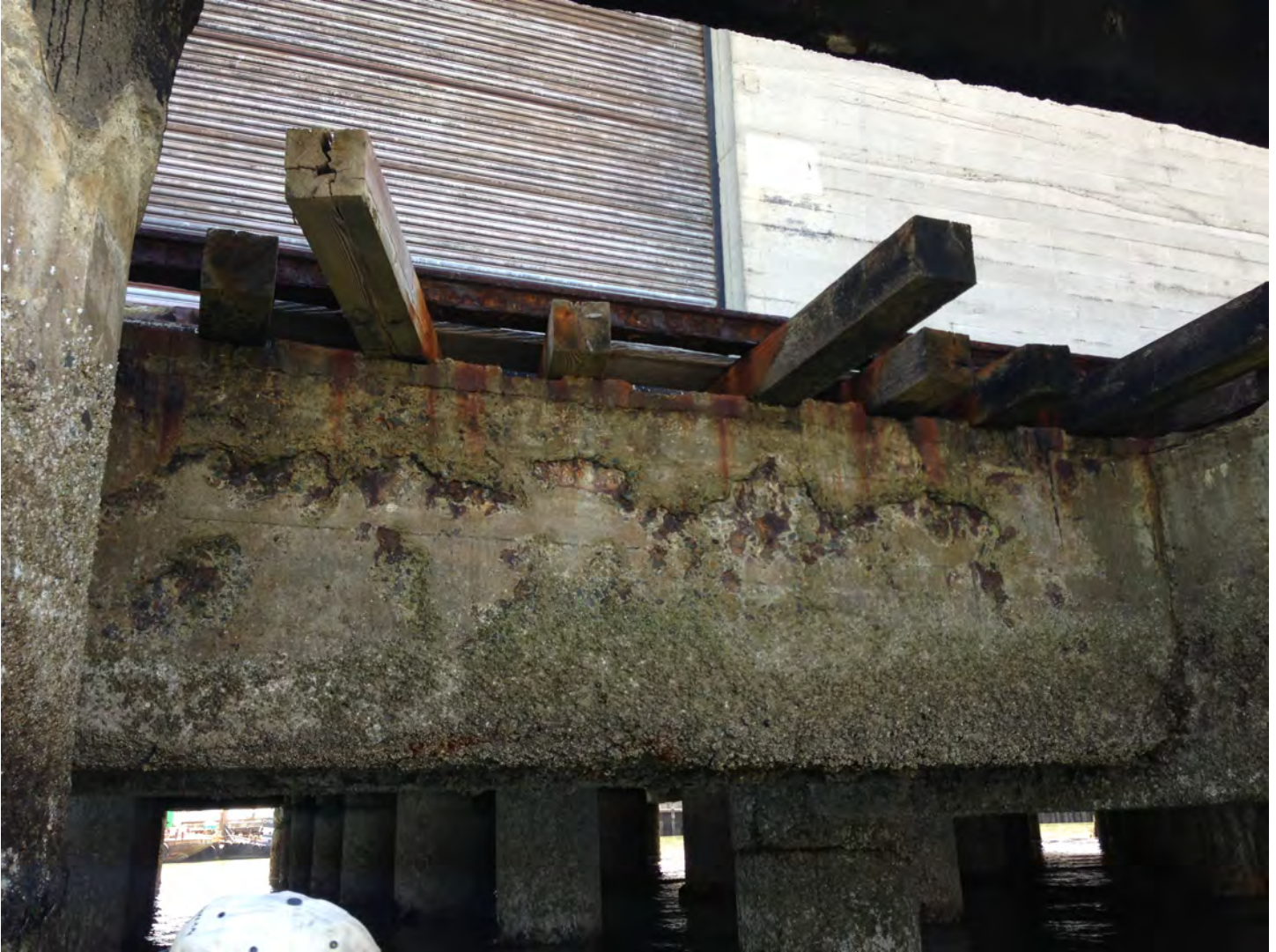
Photo 4. Hole in deck, hanging wood members
