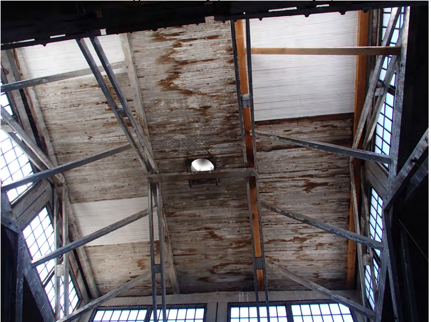
Photo 6. View of a roof pop-up area with shoring work on wood beams. Note water intrusion stains on roof sheathing
