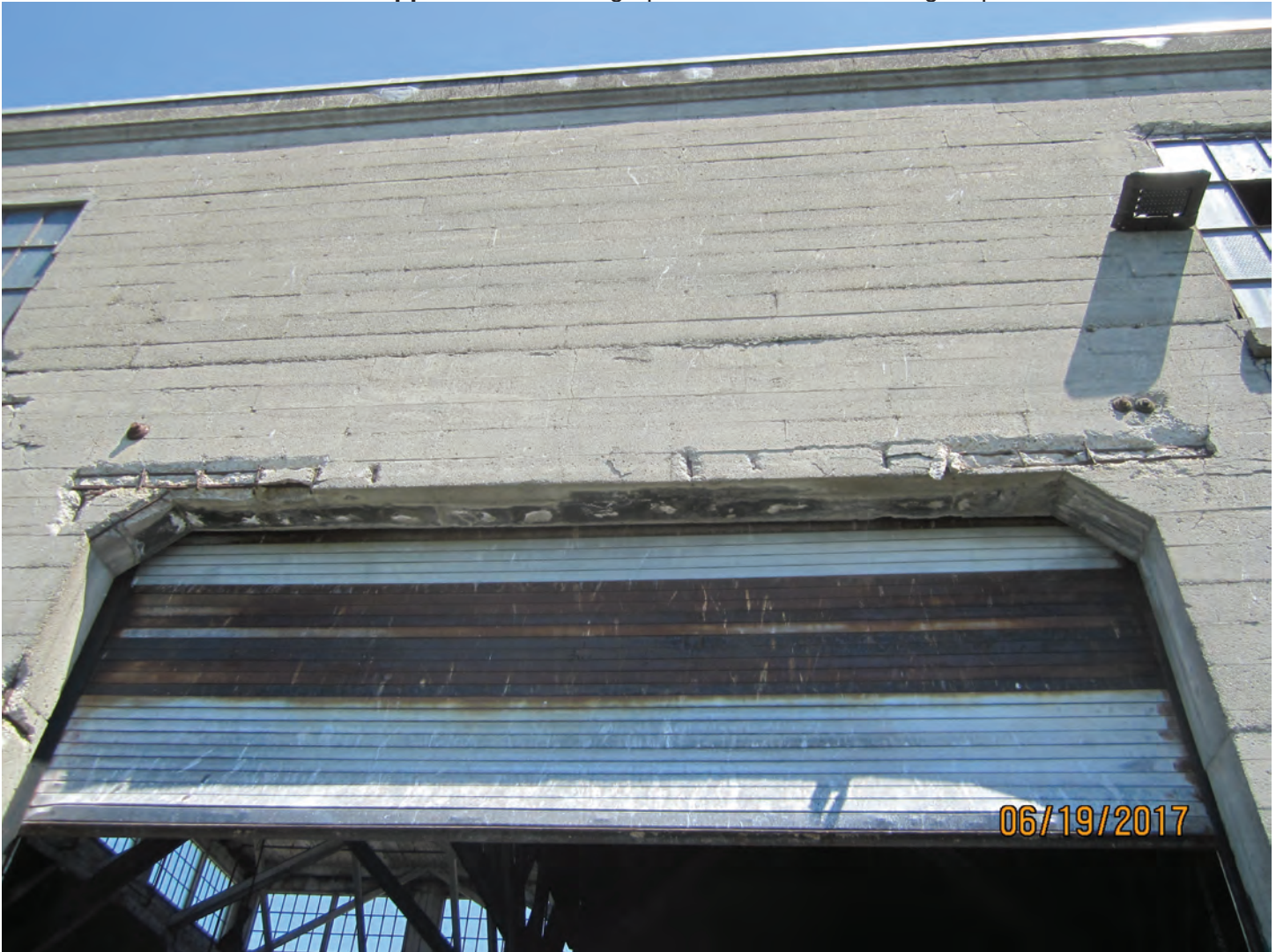
Photo 4. Spalls around roll-up door opening on north face wall. Repairs are planned as part of a future project.
