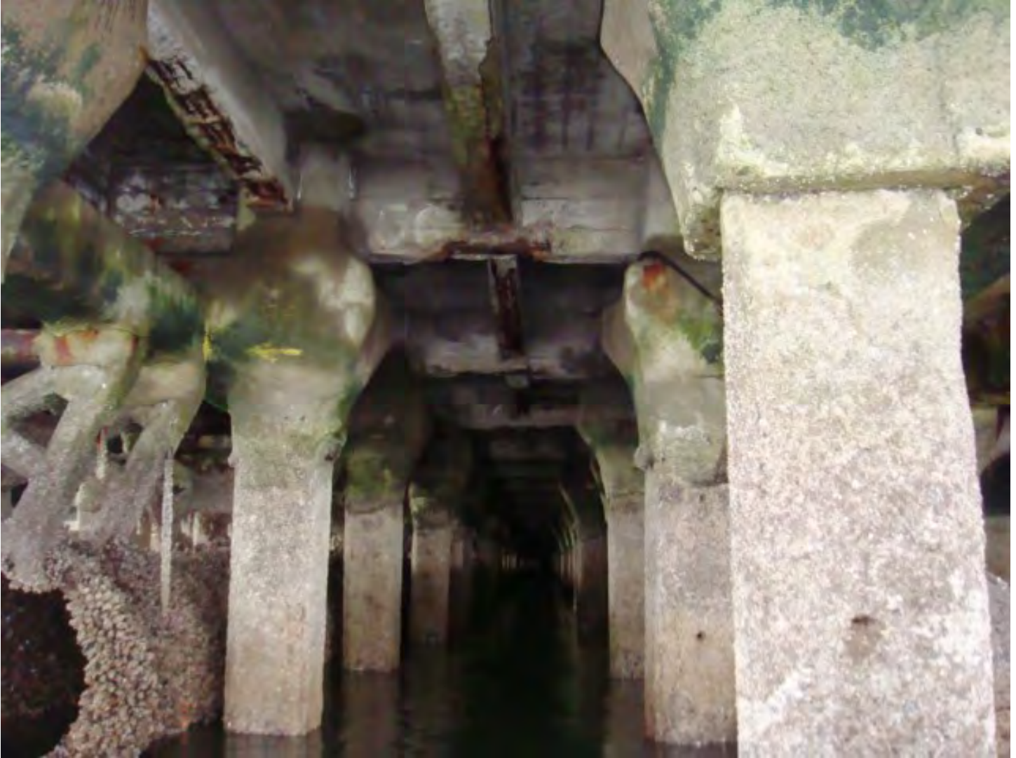
Photo 1. Spalled concrete beams and slabs above the outfalls under the Main Pier
