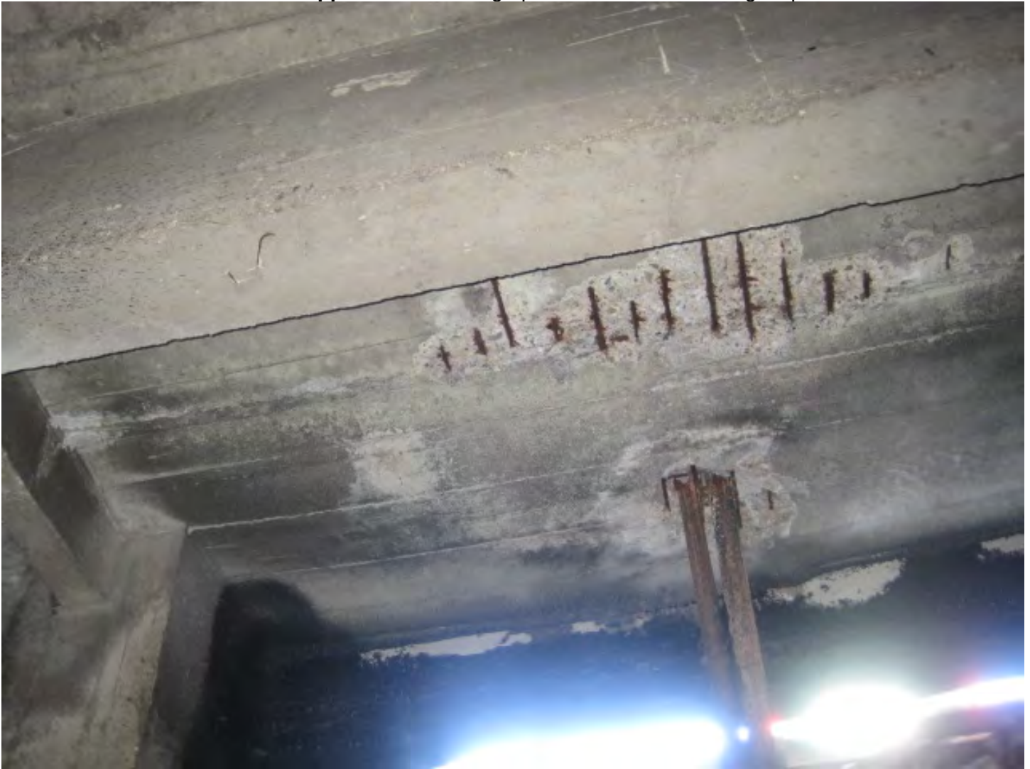
Photo 1. Spalling and corroded/exposed rebar at slab
