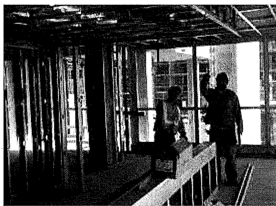
Plumbing Inspector Steven Chew inspecting an installation of sprinkler piping at 201 Folsom Street.
