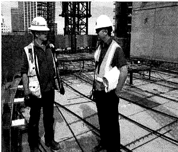
Building Inspector Fergal Clancy performs an inspection for concrete deck pour while giving direction to the sub-contractor foreman.
